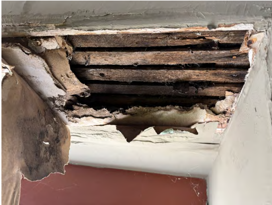
Photo 37: Deterioration from moisture ingress on third floor unoccupied space
