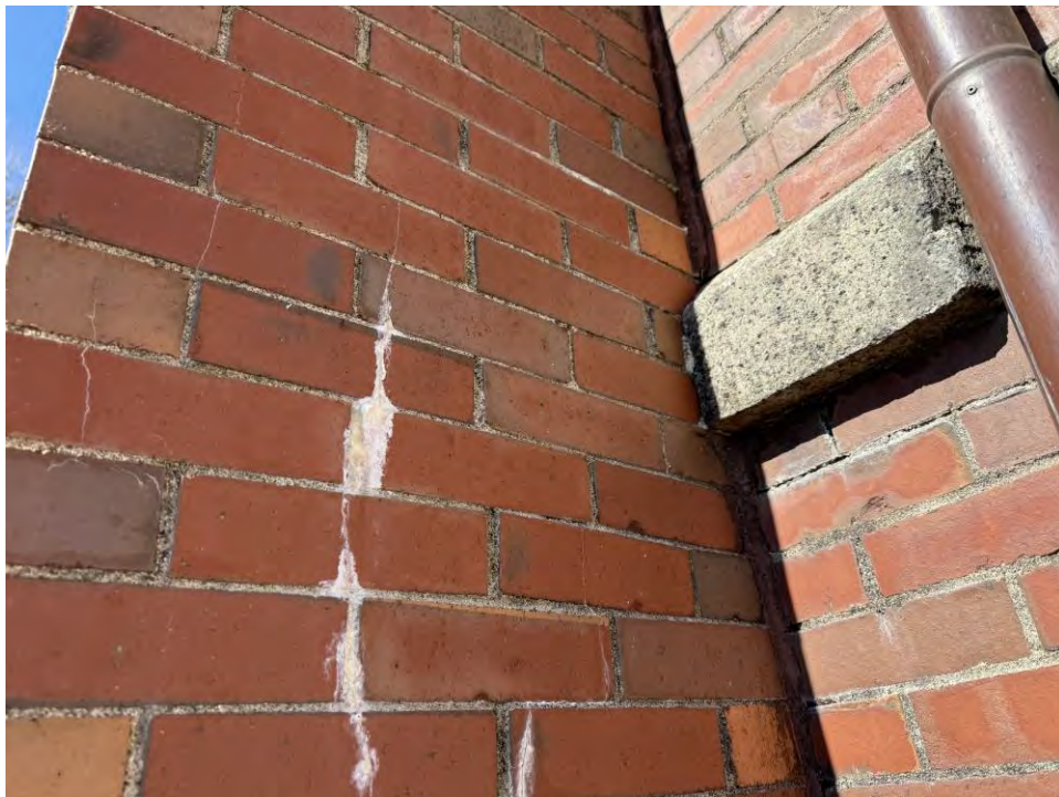
Photo 22: Efflorescence on pilaster adjacent to south elevation Cumberland Street entrance
