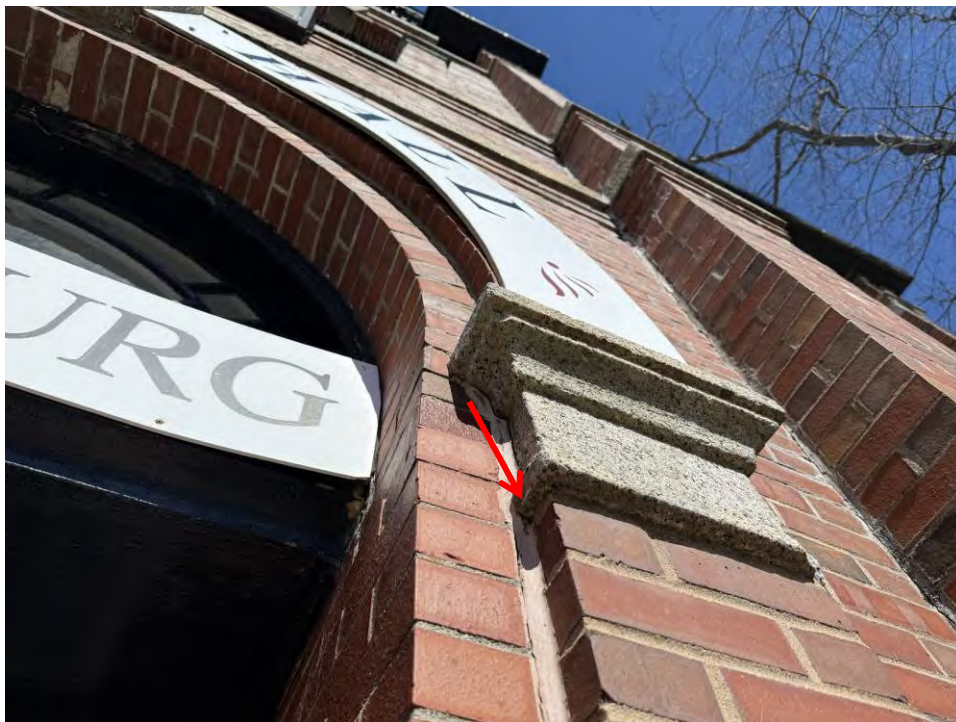
Photo 12: Sealant between different vintages of brick with cohesive tears
