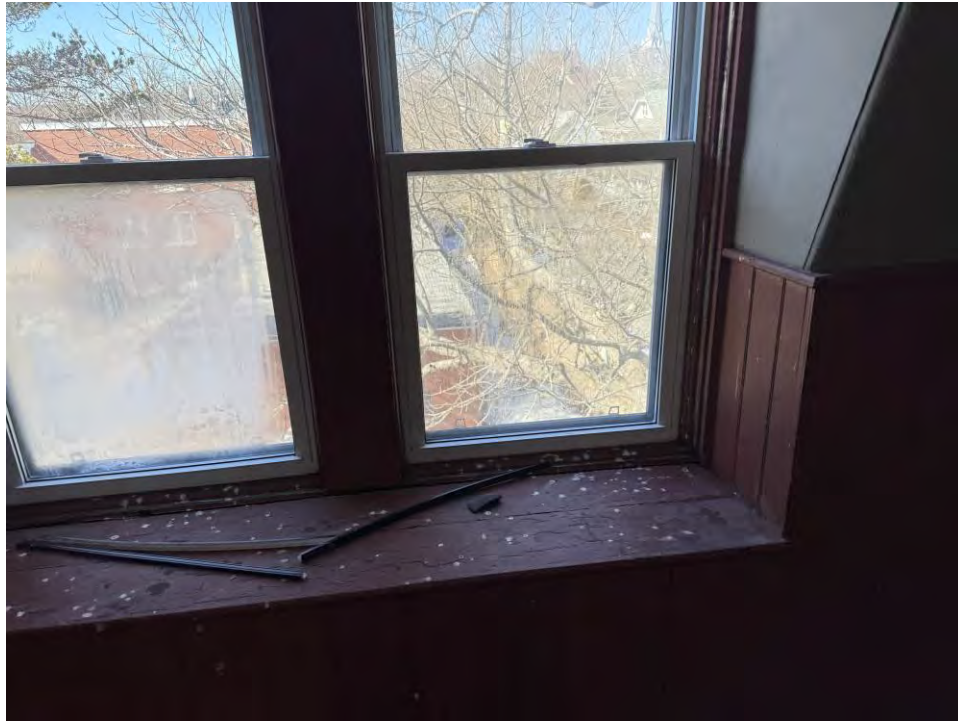
Photo 29: Failed IGUs in top floor unoccupied space
