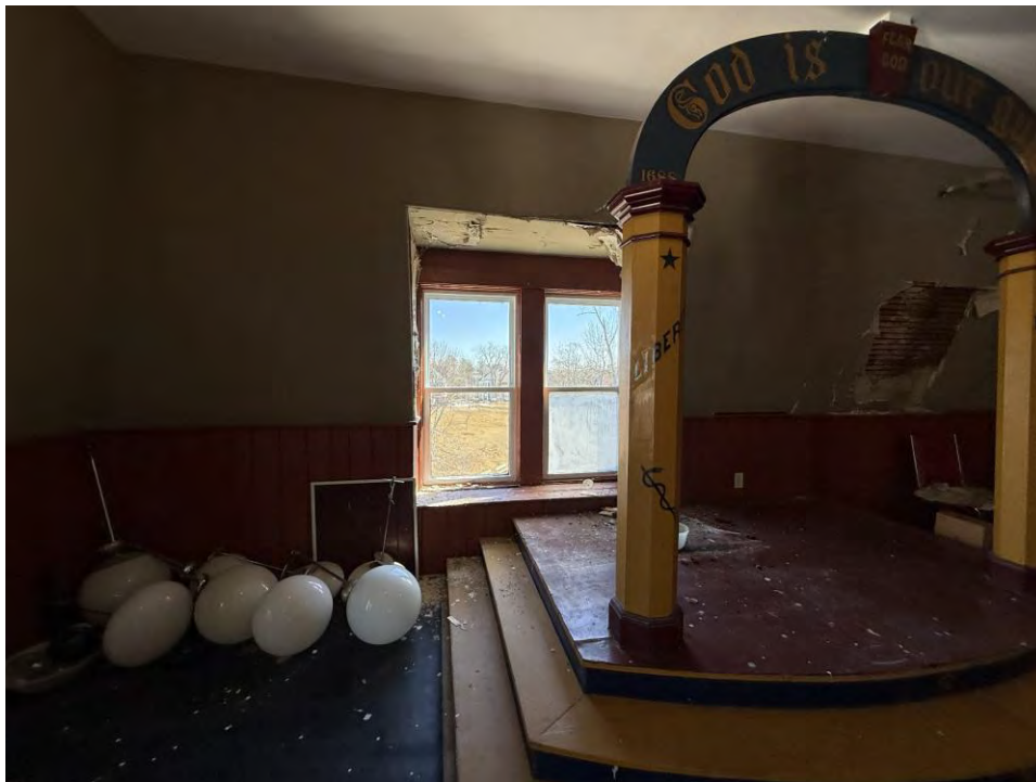
Photo 28: Newer vinyl windows in an unoccupied room on north side of third floor (typ. at four dormers)
