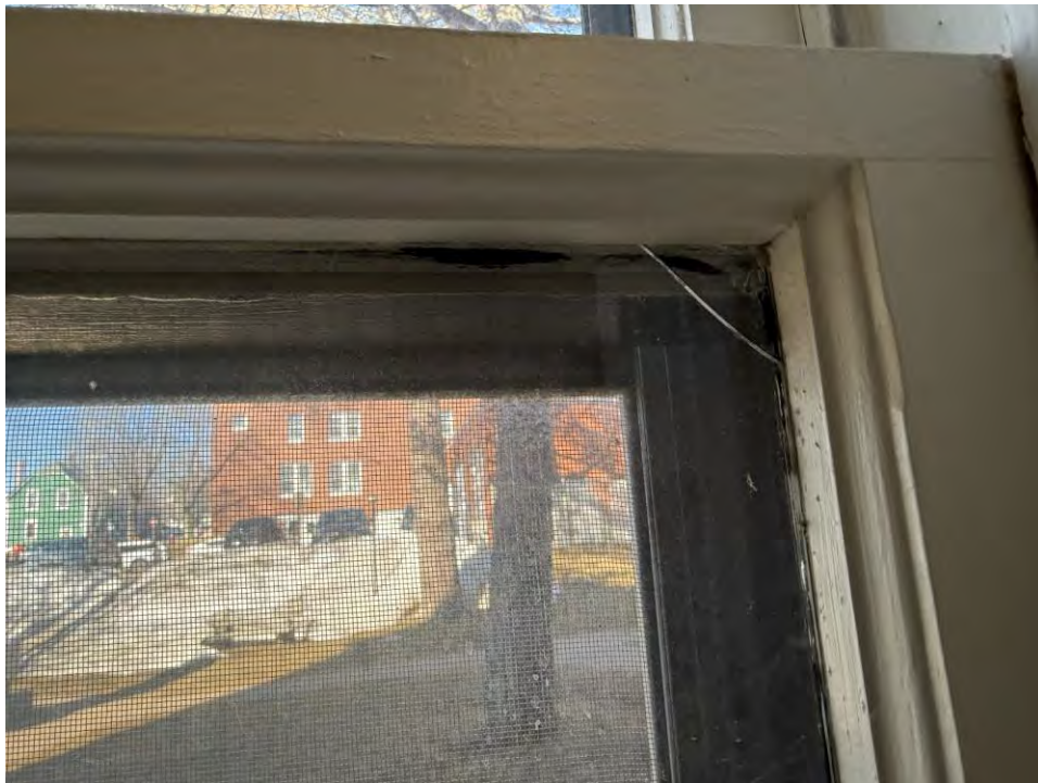
Photo 30: Cracked pane on second floor office window on west elevation
