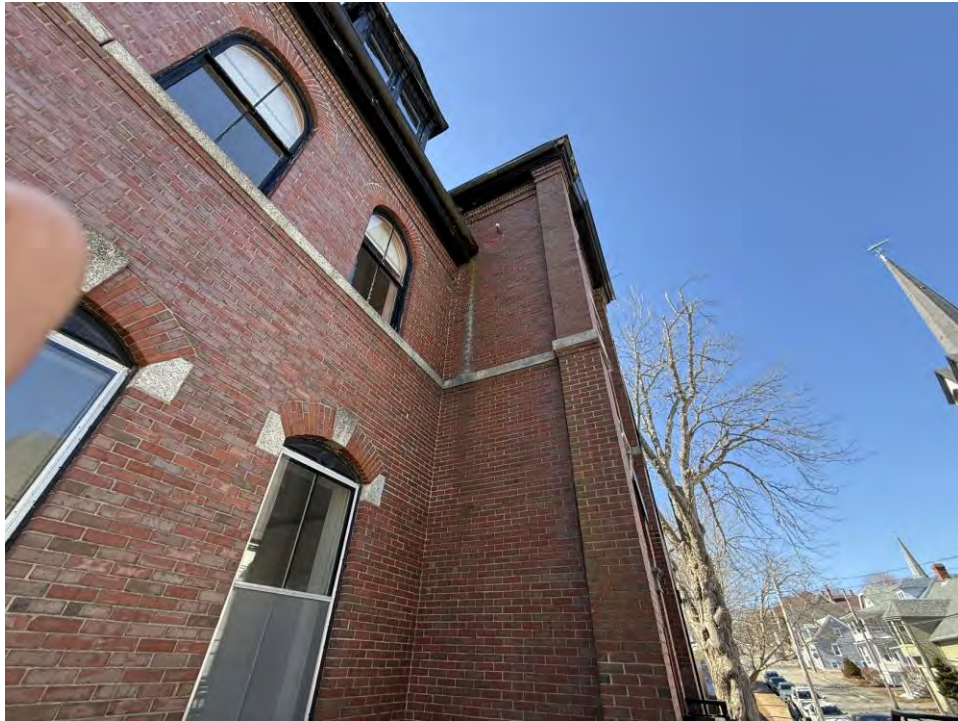
Photo 21: Overview of run-off and organics staining below gutter likely from overflow
