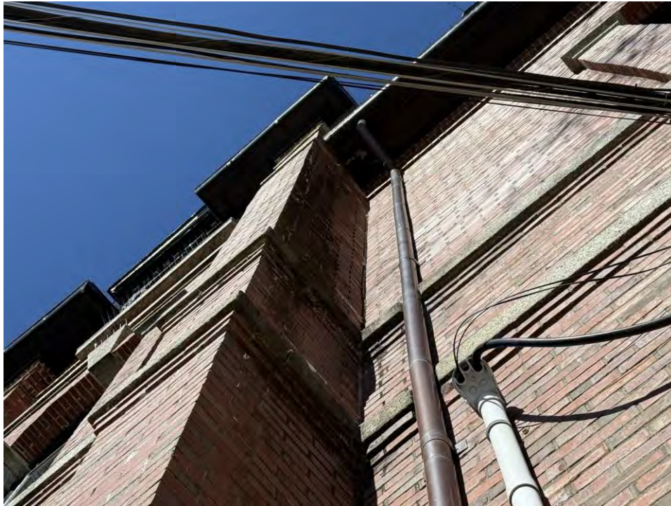
Photo 19: Overview of staining from gutter run-off on south elevation Cumberland Street entrance
