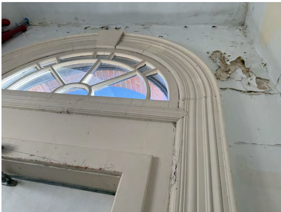
Photo 32: Moisture ingress deterioration above east elevation entrance
