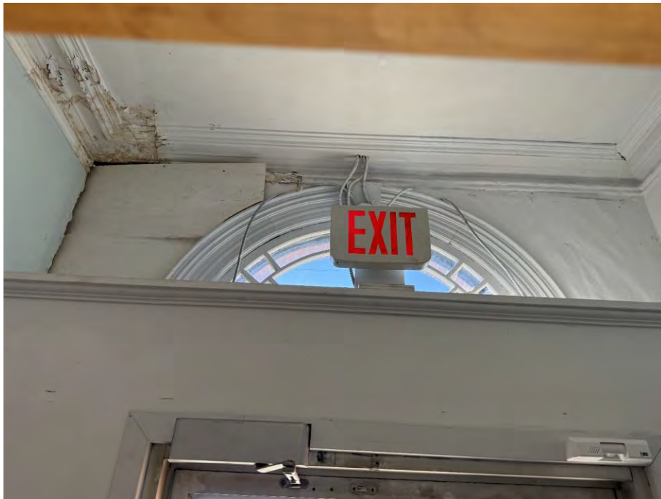
Photo 31: Moisture ingress deterioration above south elevation Cumberland Street entrance
