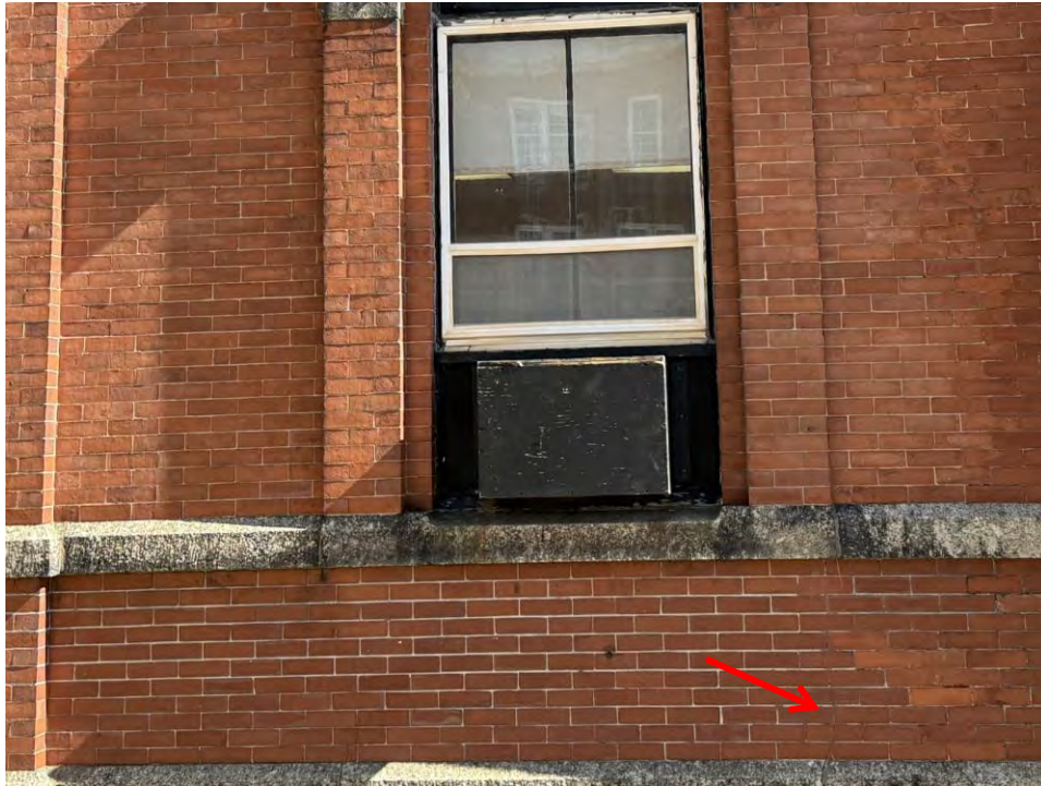
Photo 15: Close up of brick cracking and deterioration along west elevation
