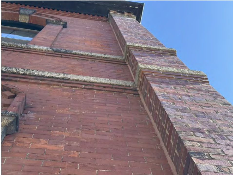
Photo 17: Overview of brick face spalling near southwest corner pilaster on west elevation
