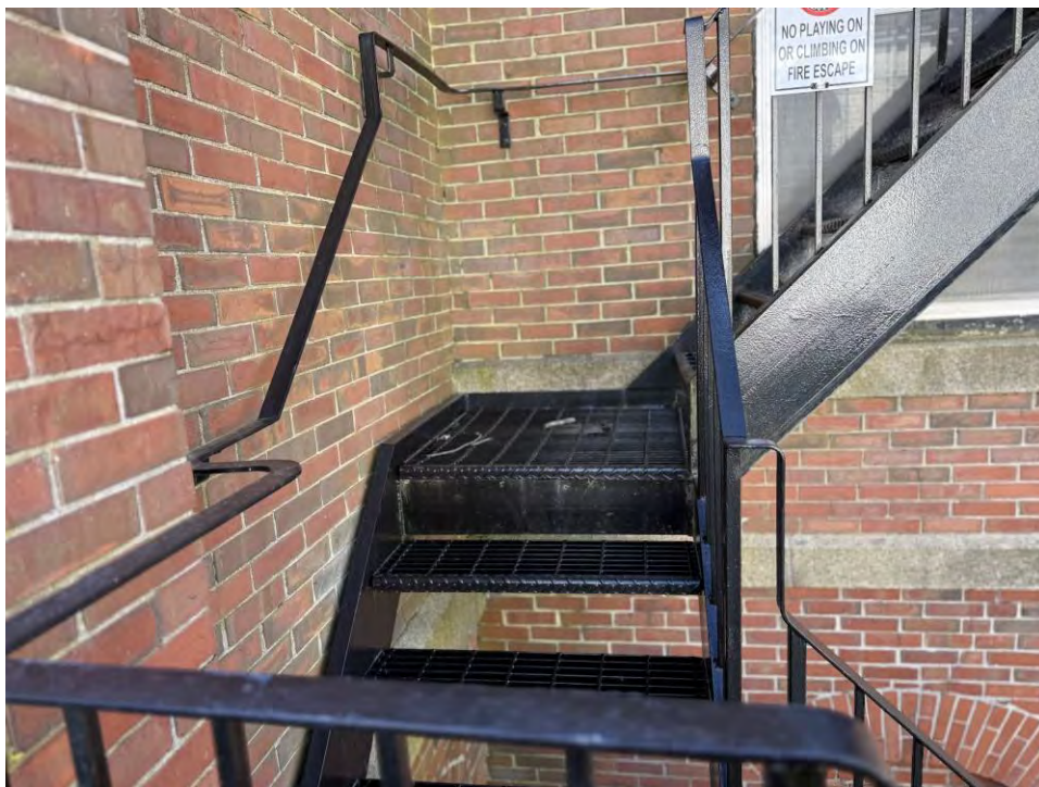
Photo 20: Overview of organics staining below fire escape stairs on north elevation Townsend Street entrance
