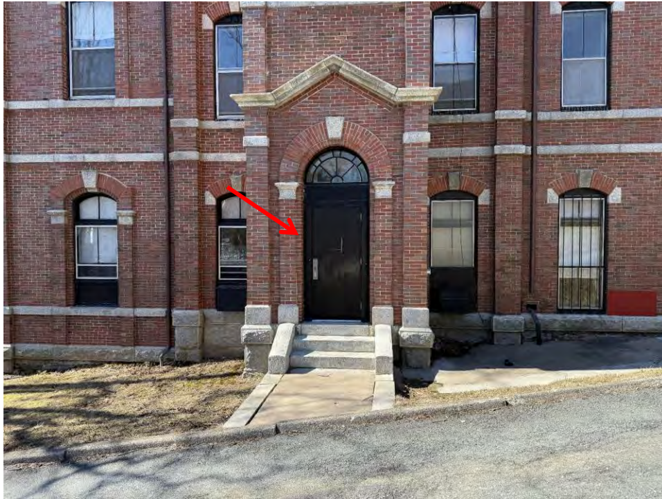
Photo 11: Existing brick repair areas near east elevation entrance
