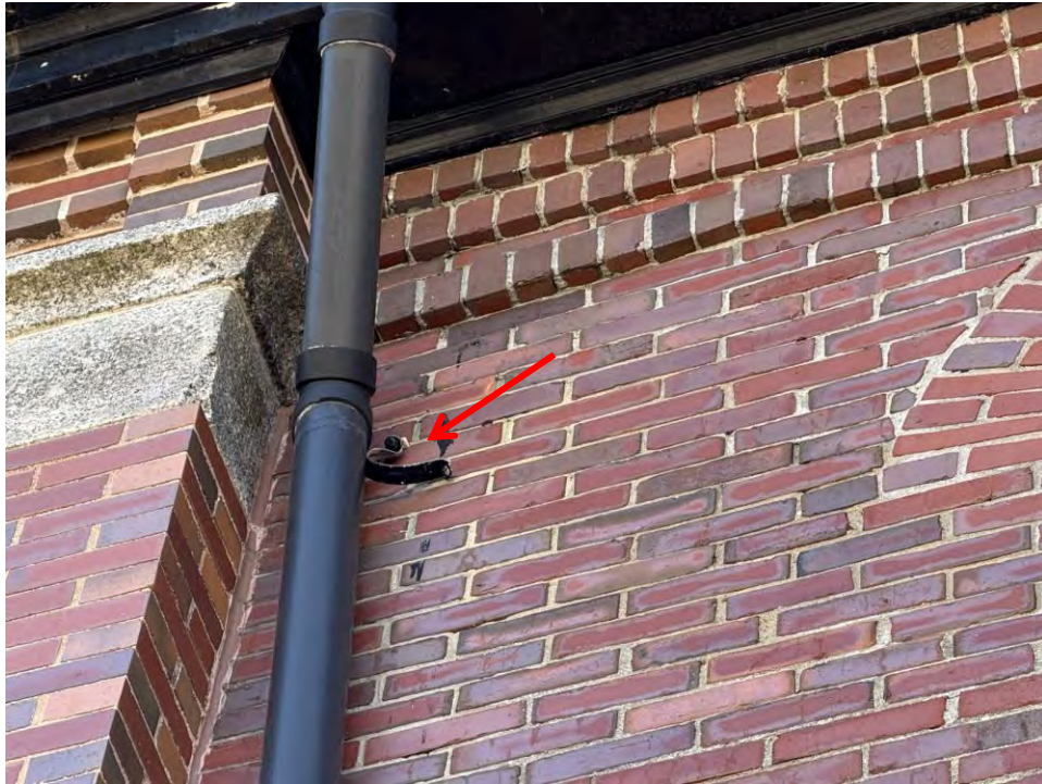
Photo 7: Pulled/failed anchor for downspout strapping
