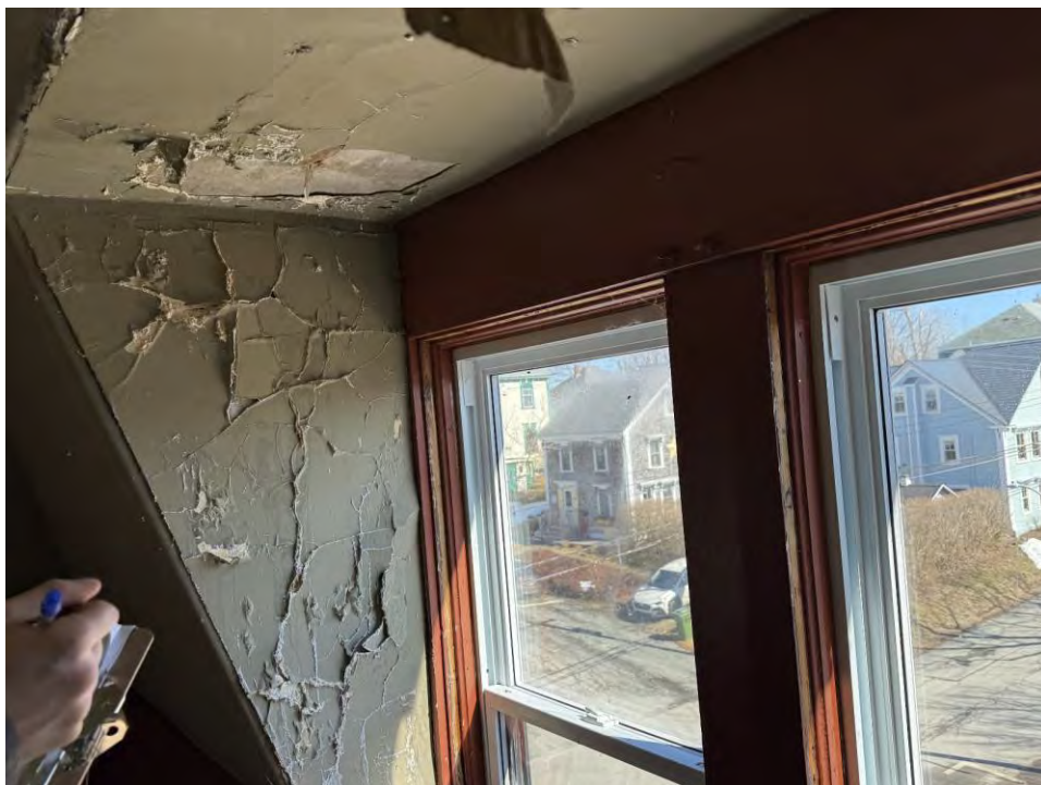
Photo 34: Deterioration from moisture ingress on third floor unoccupied space
