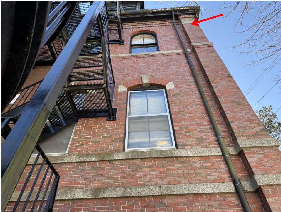
Photo 23: Slight bow at top of northwest corner pilaster
