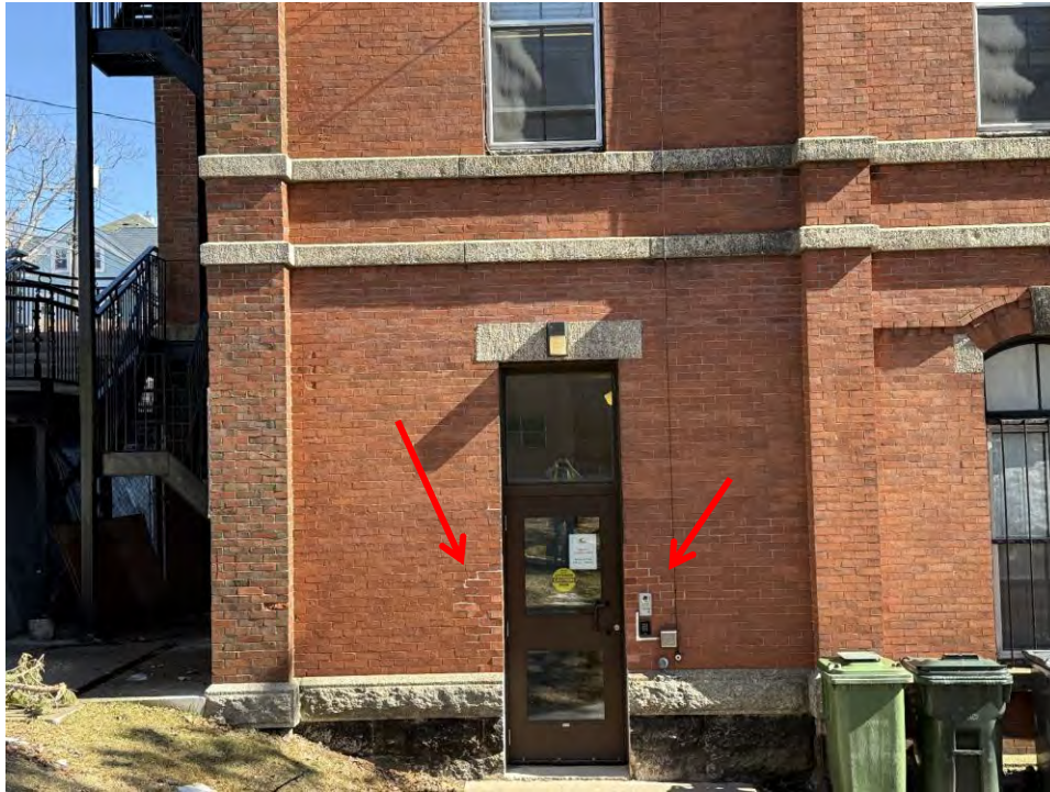
Photo 9: Existing brick repair areas near west elevation entrance
