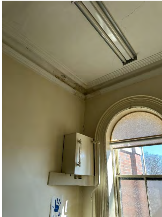
Photo 39: Deterioration from moisture ingress on third floor
