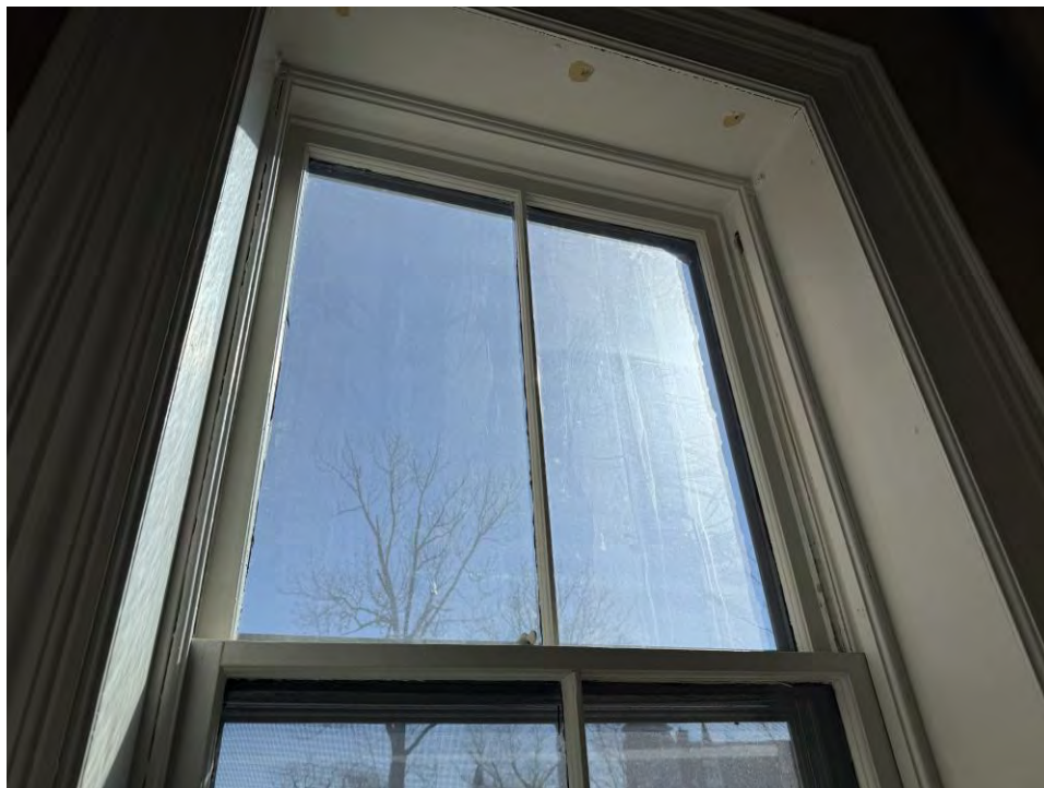
Photo 26: Visual evidence of water runoff/dripping on interior face of windows
