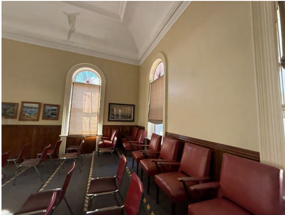
Photo 38: Deterioration from moisture ingress on second floor in Council chambers
