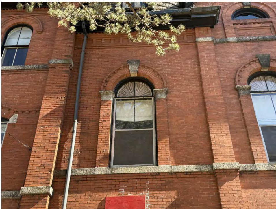
Photo 16: Overview of mortar joint deterioration in vicinity of west elevation downspout
