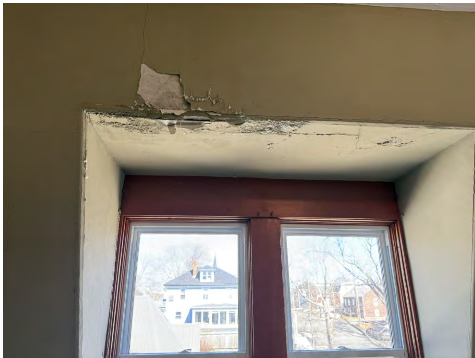
Photo 36: Deterioration from moisture ingress at dormer window on third floor unoccupied space
