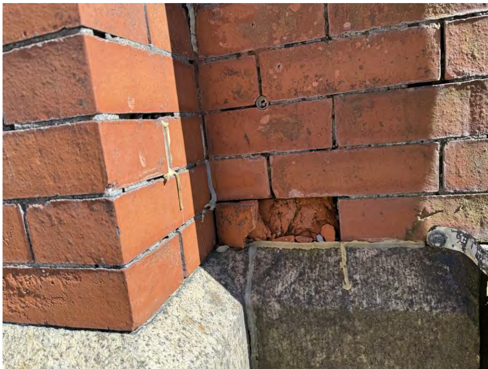
Photo 18: Closeup of brick-and-mortar joint deterioration
