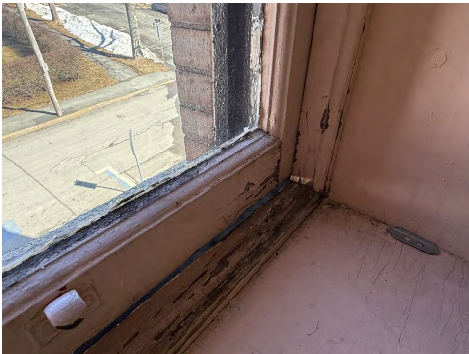
Photo 24: Peeling paint and deterioration on wood window, likely from condensation
