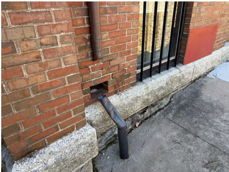
Photo 8: Copper downspout (note discontinuity)
