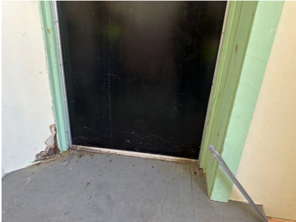
Photo 33: Moisture ingress deterioration at third storey fire escape door
