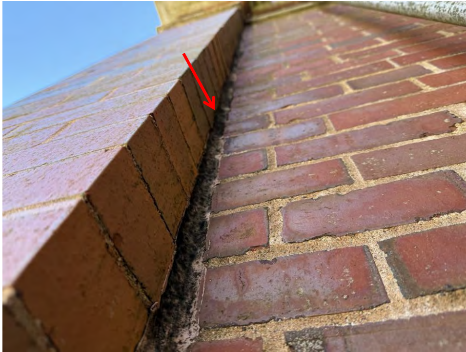
Photo 13: Sealant between different vintages of brick with crazing and organics
