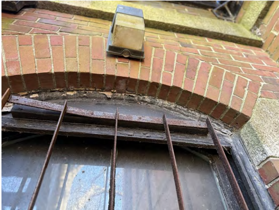
Photo 25: Peeling paint and deterioration of exterior wood detailing above retrofit vinyl window
