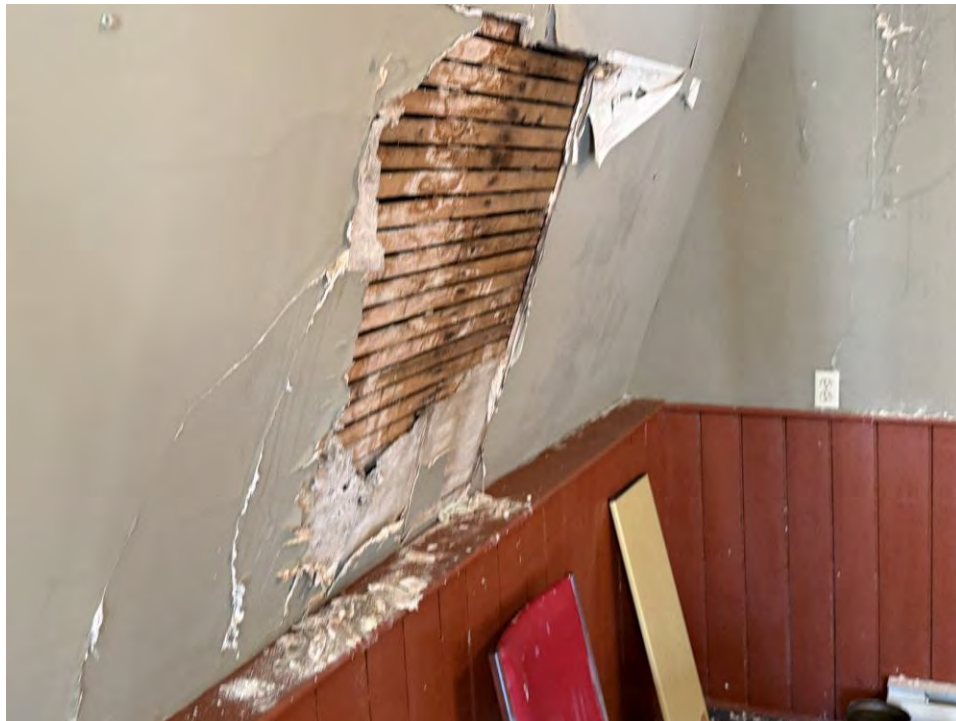
Photo 35: Deterioration from moisture ingress on third floor unoccupied space
