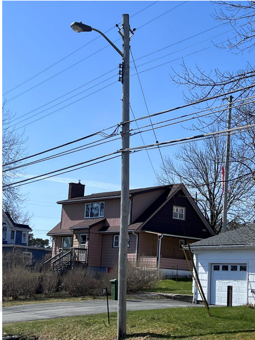
Figure 2: High Pressure Sodium Fixture Installed in the Overhead Line Primary Zone
