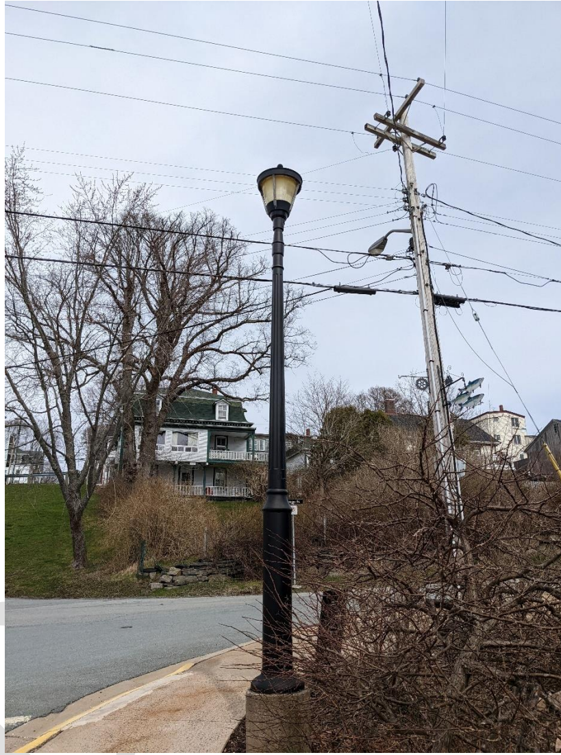
Figure 7: Historic Lighting Fixture Style 2 Installed on a Custom Pole
