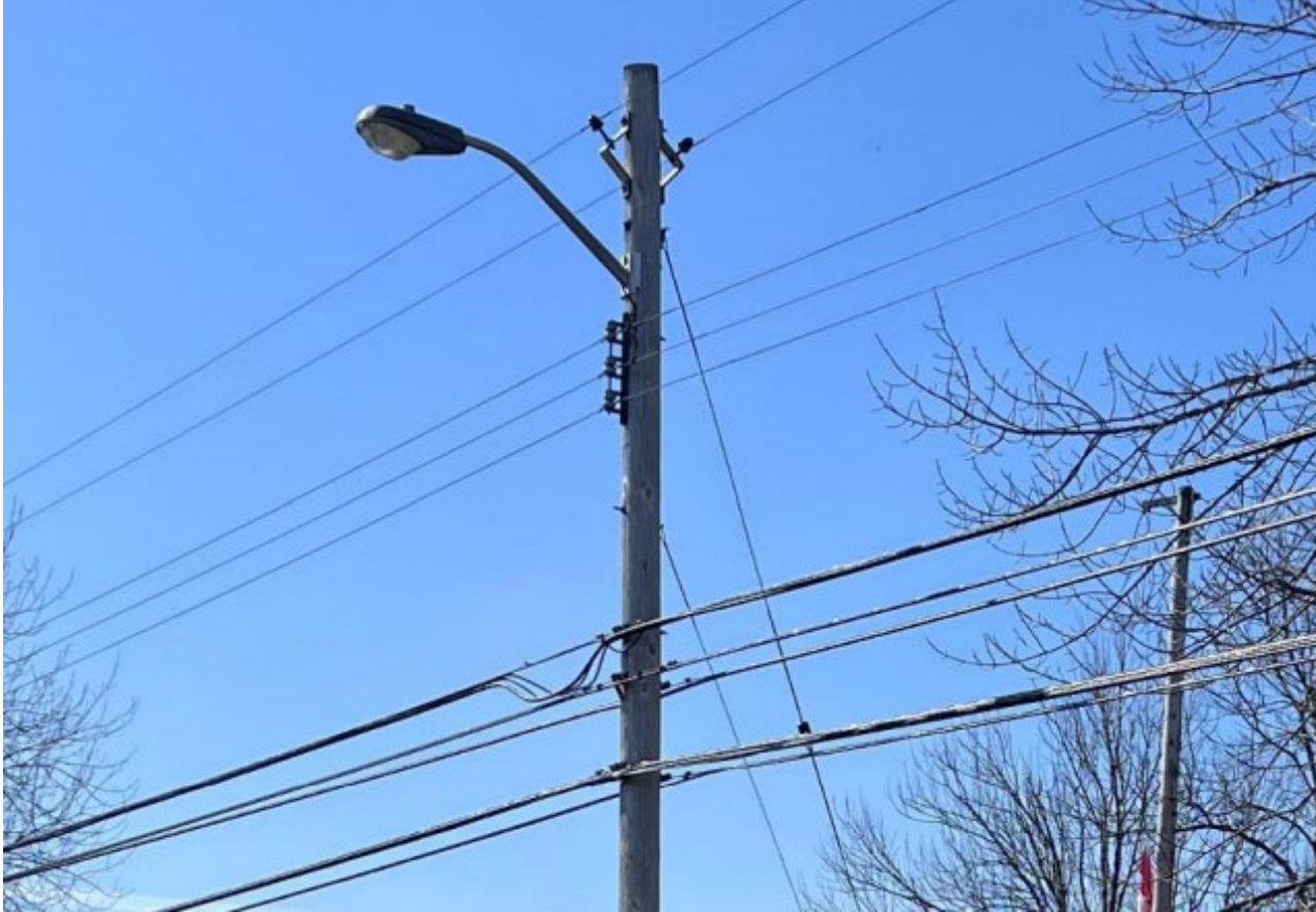
High Pressure Sodium Fixture Installed in the Overhead Line High Voltage Zone
