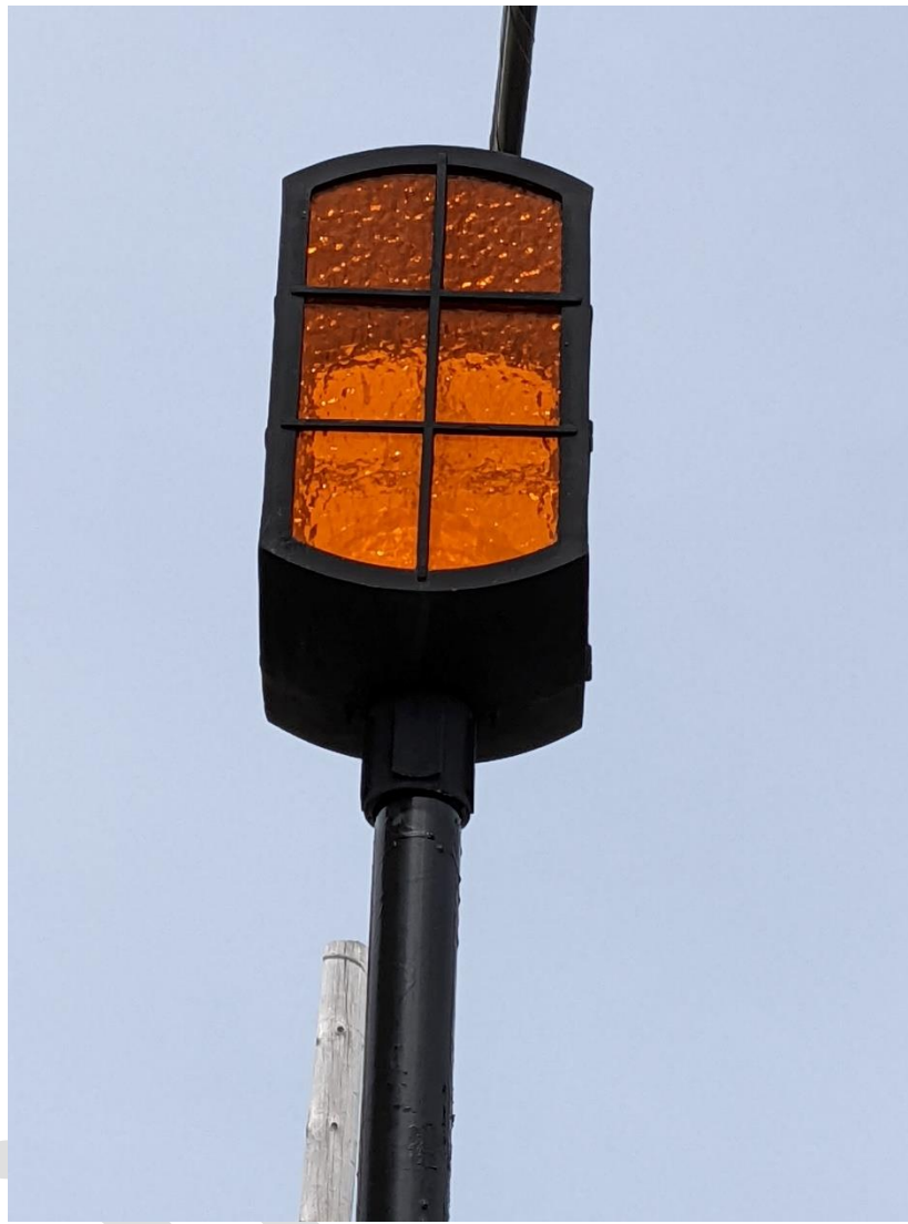
Figure 9: Historic Lighting Fixture Style 4 Dual Fixture Installed on a Custom Pole
