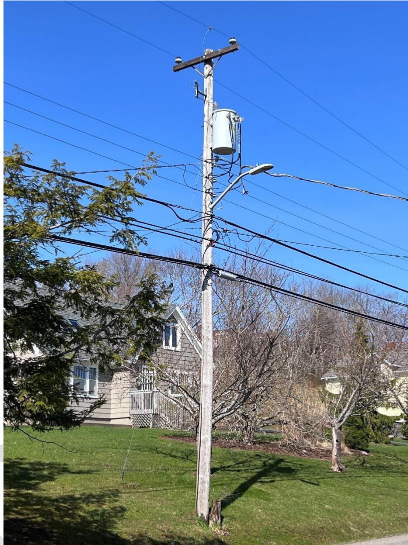
Figure 3: LED Fixture Installed below the Overhead Line Primary Zone
