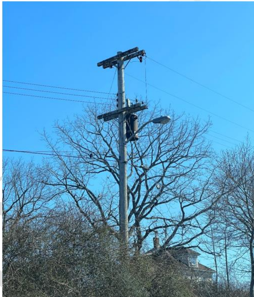
Figure 1: High Pressure Sodium Fixture Installed below the Overhead Line Primary Zone
