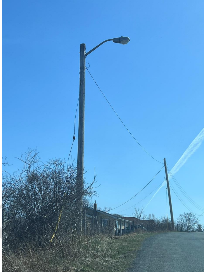
Figure 4: High Pressure Sodium Fixture Installed on a Secondary Conductor Utility Pole
