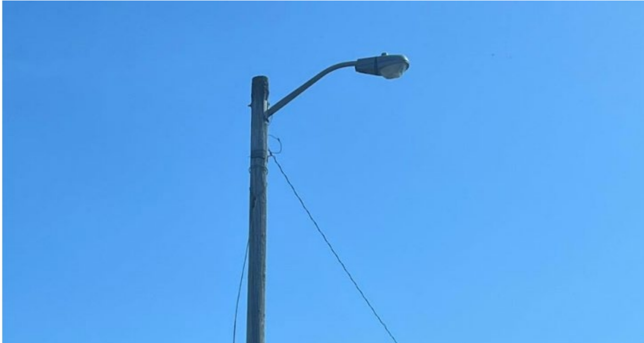
High Pressure Sodium Fixture Installed on a Low Voltage Pole
