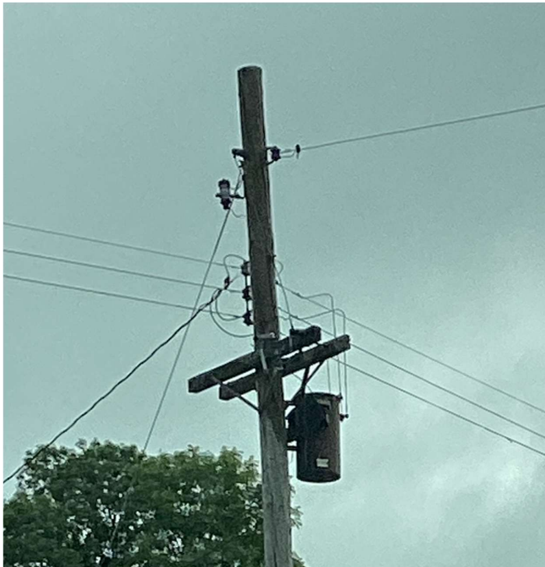
Figure 1: Underslung Transformer with potential PCB's
