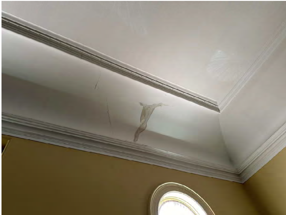
Photo 51: Deterioration from moisture ingress on second floor in Council chambers
