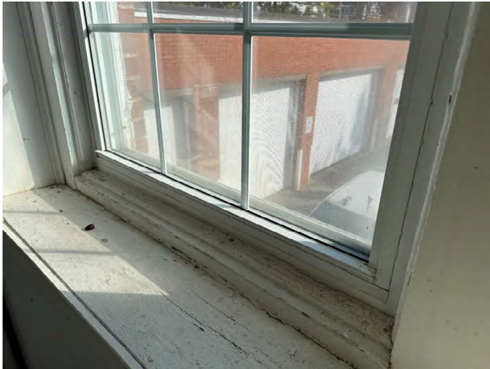
Photo 12: Interior close up of newer vinyl window (typ. throughout building) set in original wood frame in fair to poor condition
