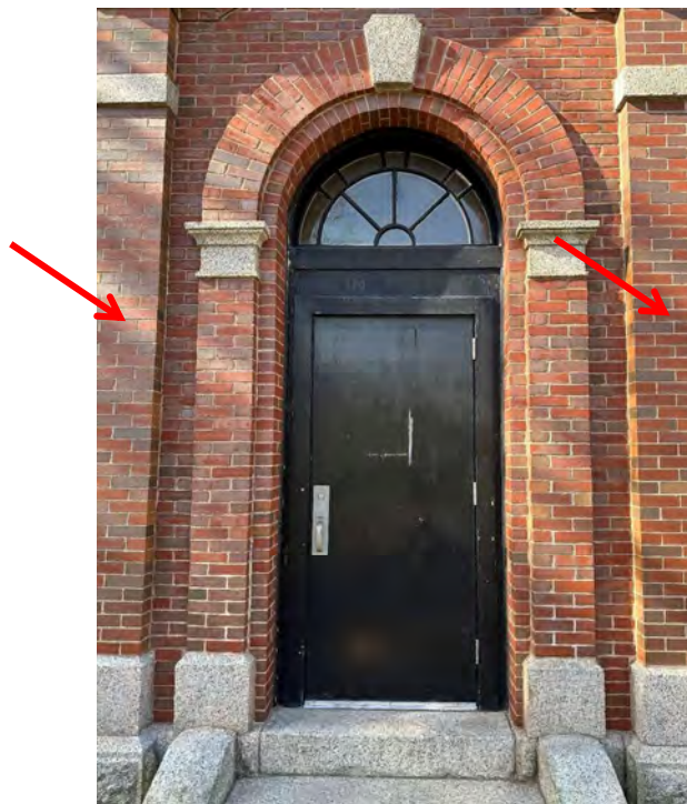
Photo 20: Existing brick repair areas near east elevation entrance
