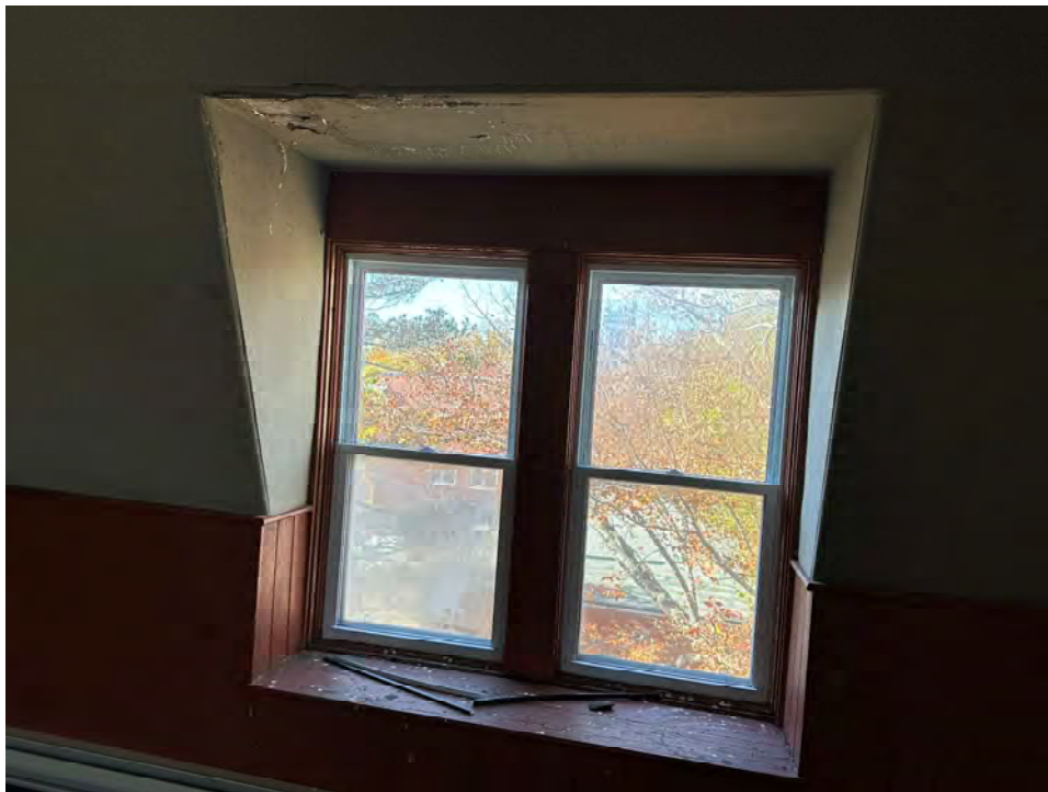
Photo 38: Newer vinyl windows in an unoccupied room on north side of third floor (typ. at four dormers)
