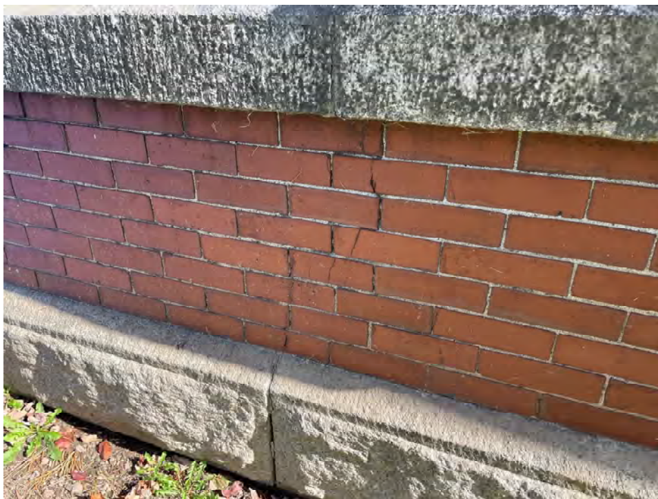
Photo 24: Close up of brick cracking and deterioration along west elevation
