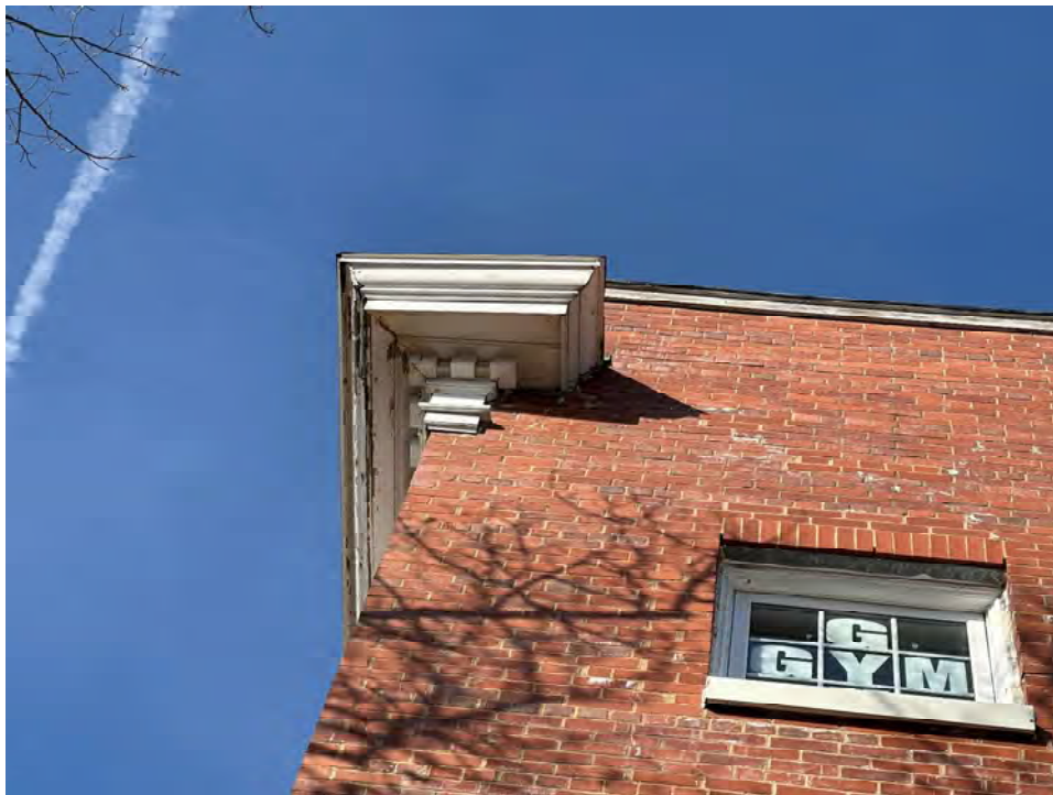
Photo 17: Failing paint finish and deterioration on underside of wood cornice at southeast corner
