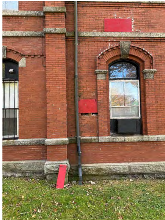
Photo 11: PVC downspout terminating below-grade
