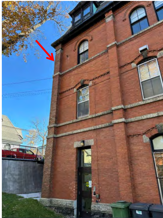
Photo 31: Slight bow at top of northwest corner pilaster
