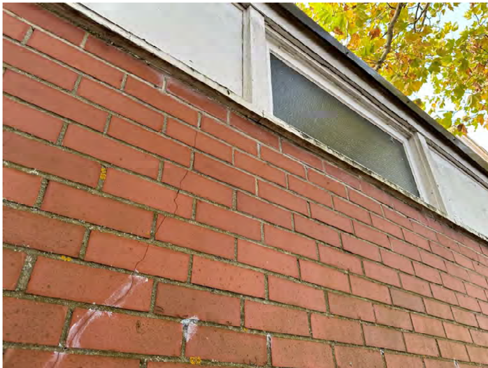
Photo 6: Brick cracking on north elevation
