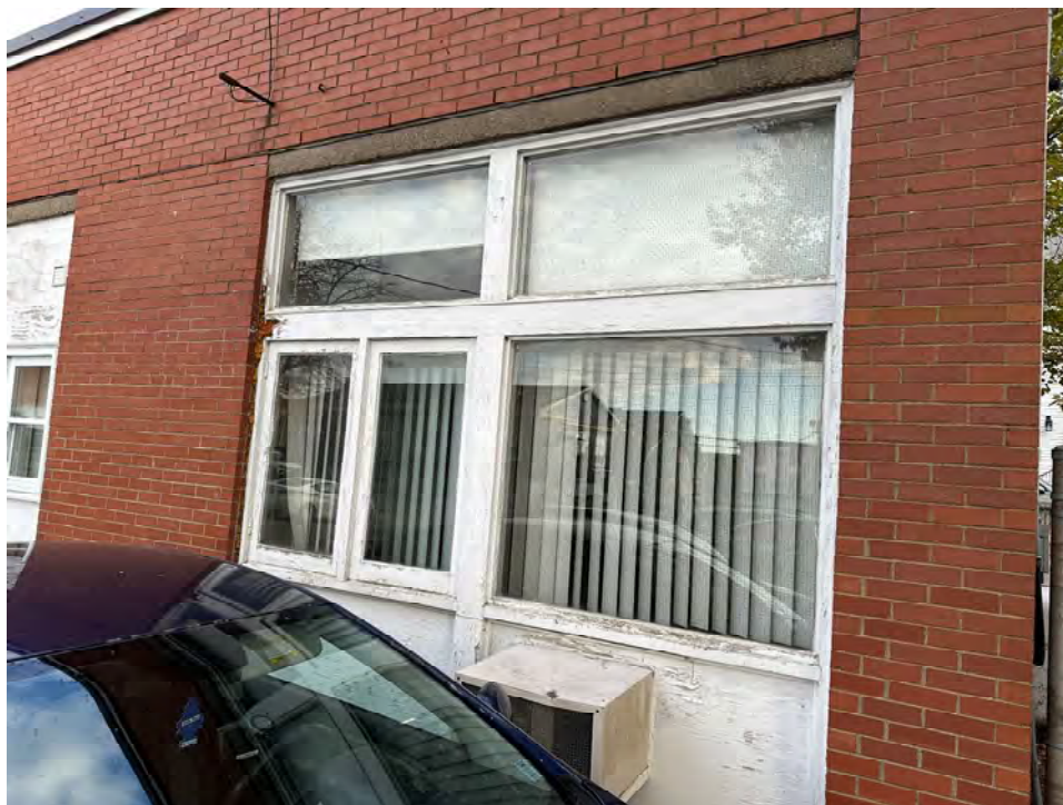
Photo 16: Deteriorated window unit on south elevation
