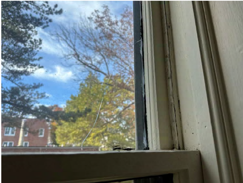
Photo 39: Cracked pane on second floor office window on west elevation
