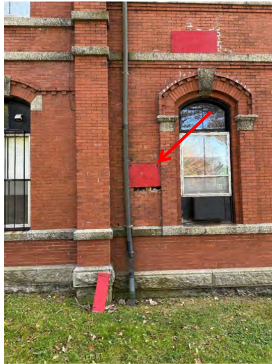
Photo 33: Exploratory opening on west elevation by others and reopened for RJC review
