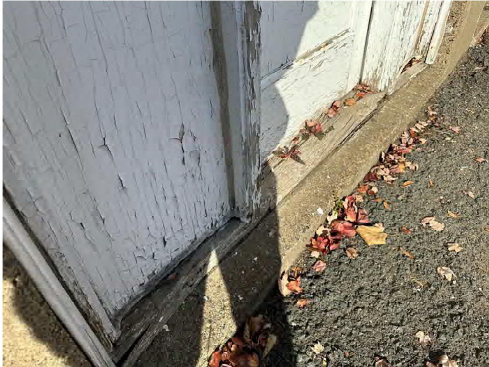
Photo 10: Close up of east elevation door with deteriorated wood threshold and failing paint finish
