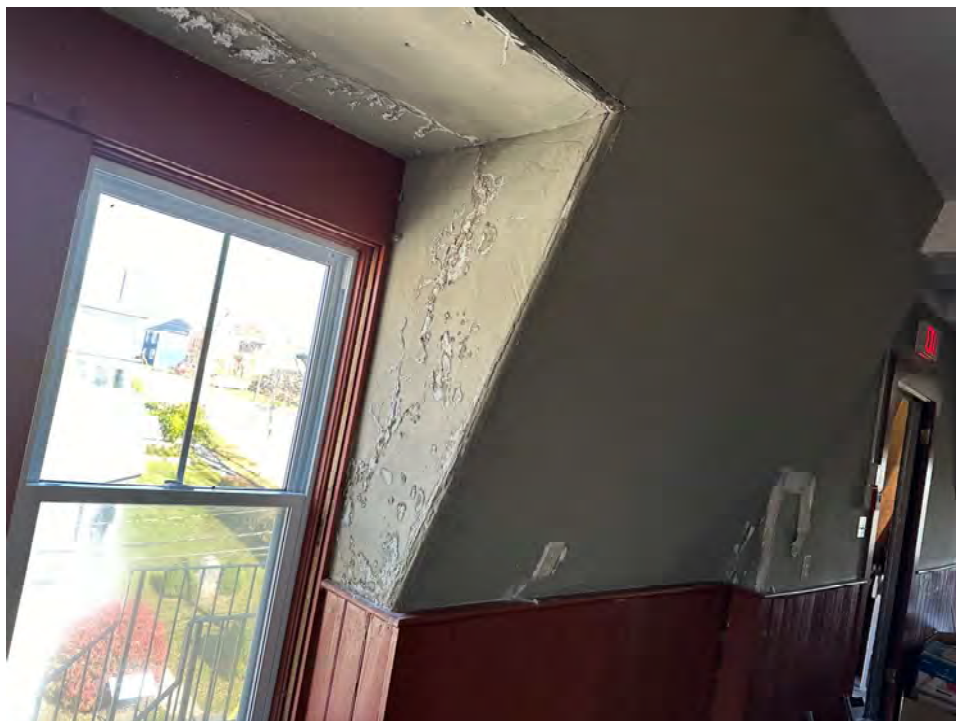
Photo 50: Deterioration from moisture ingress at dormer window on third floor unoccupied space
