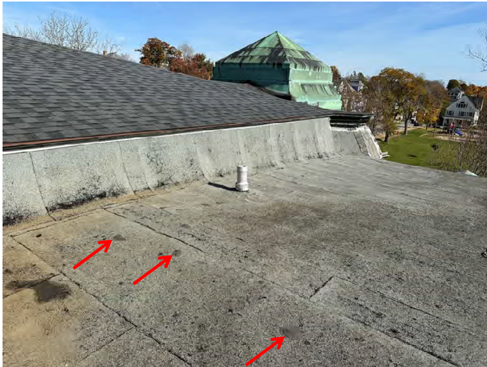
Photo 7: Newer asphalt shingle roofing, modified bitumen sheet membrane, copper roof projection. Note localized liquid-applied patch repairs
