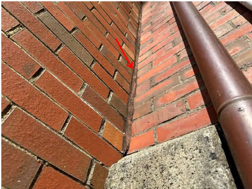
Photo 22: Sealant between different vintages of brick with crazing
