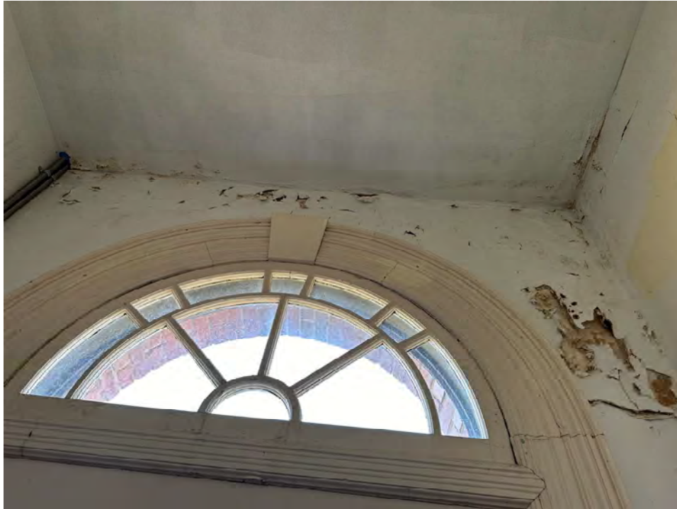
Photo 41: Moisture ingress deterioration above east elevation entrance
