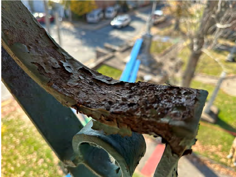
Photo 15: Peeling paint and corrosion on ornamental steel brackets
