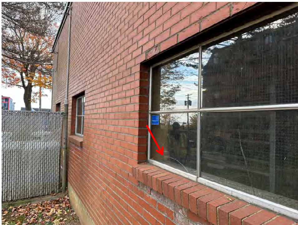
Photo 18: Cracked pane on east elevation aluminum-framed window with wired glass
