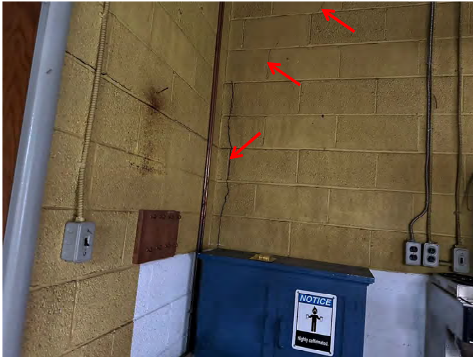
Photo 13: CMU cracking on north elevation wall
