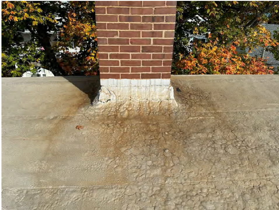
Photo 16: Alligator cracking on roofing membrane telescoping through the coating at north chimney
