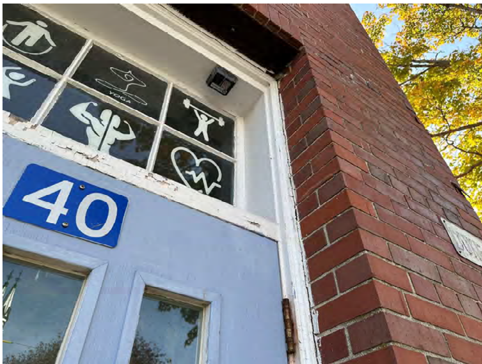
Photo 11: Close up of west elevation door with failing paint finish near southwest corner of building
