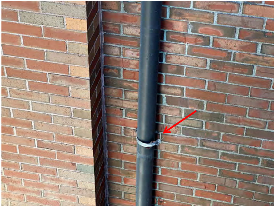
Photo 17: Pulled/failed anchor for downspout strapping
