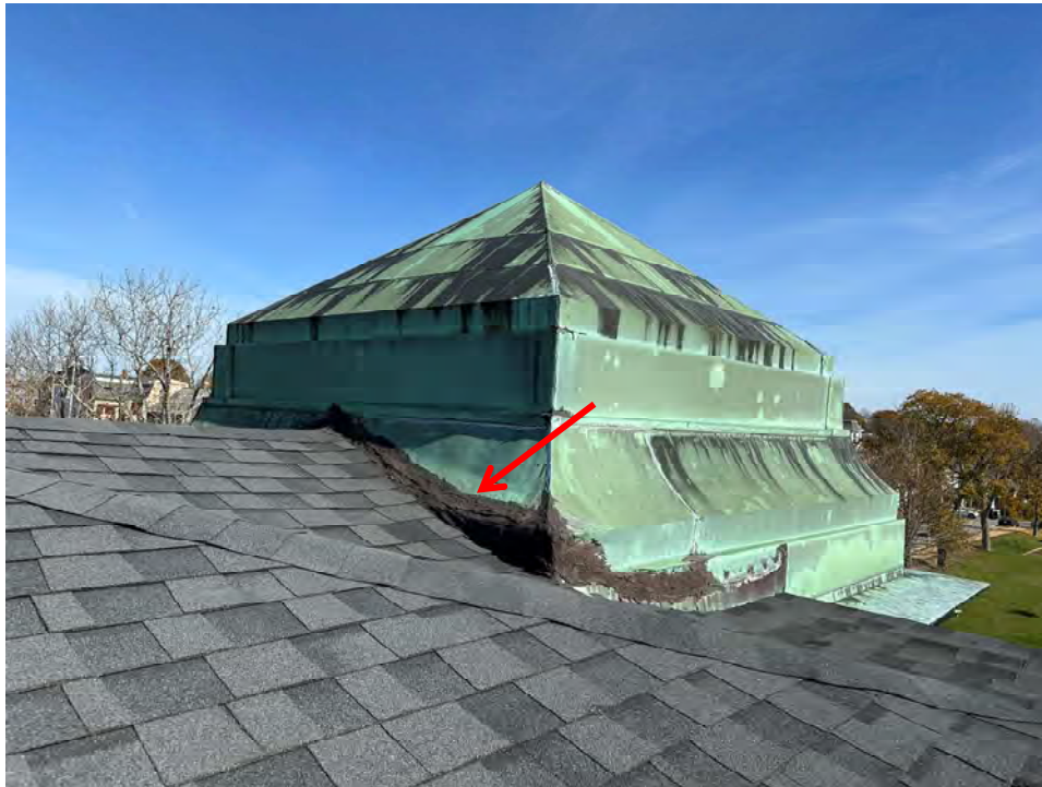
Photo 13: Roofing mastic tie-in in poor condition at transition between asphalt shingles and copper
