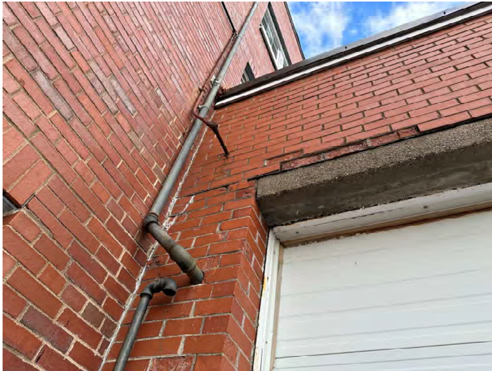
Photo 9: Brick deterioration on south elevation solid brick pier and above concrete projection/lintel from likely moisture accumulation and unsealed penetrations
