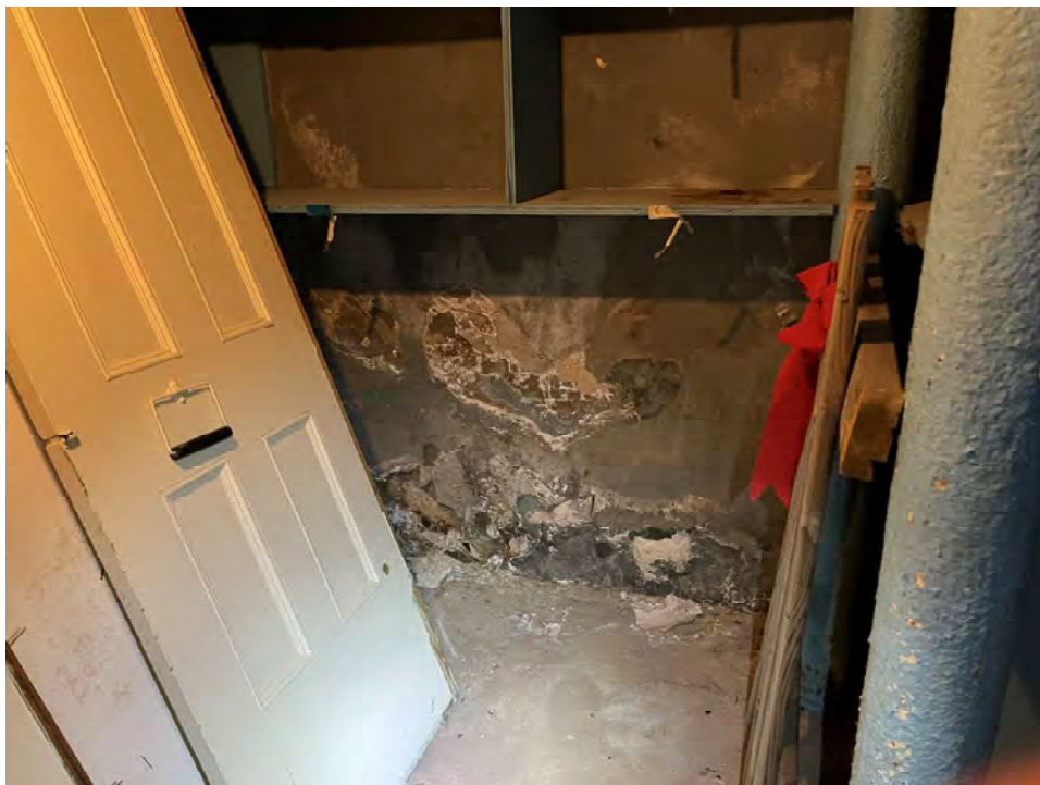
Photo 44: Deteriorated parging material on stone foundation wall
