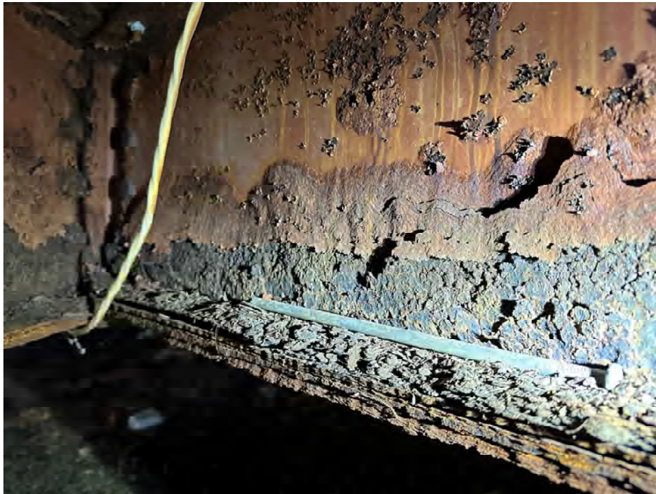
Photo 5: Corrosion and expansive corrosion by-products on beam flange
