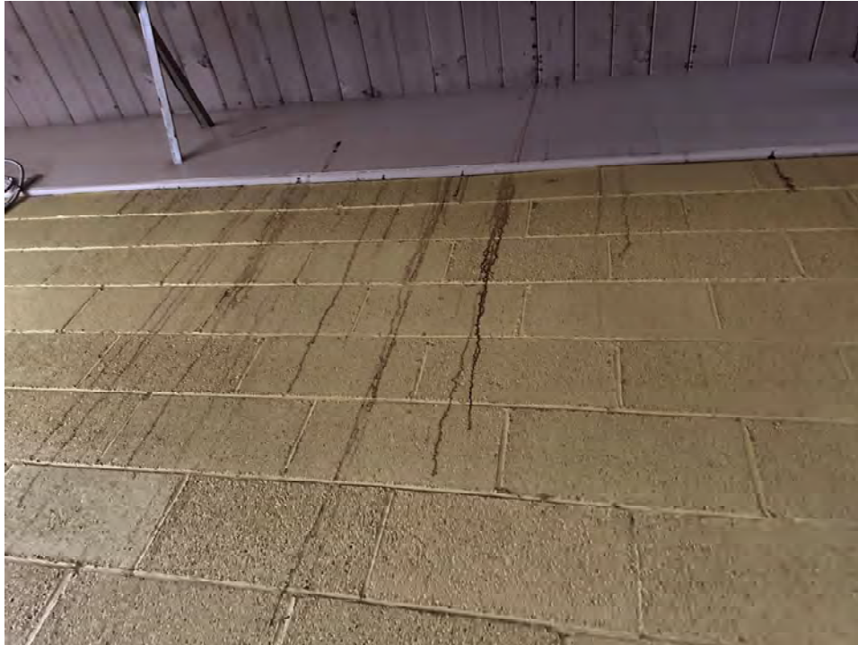
Photo 21: Indications of roof leakage on interior wall surface
