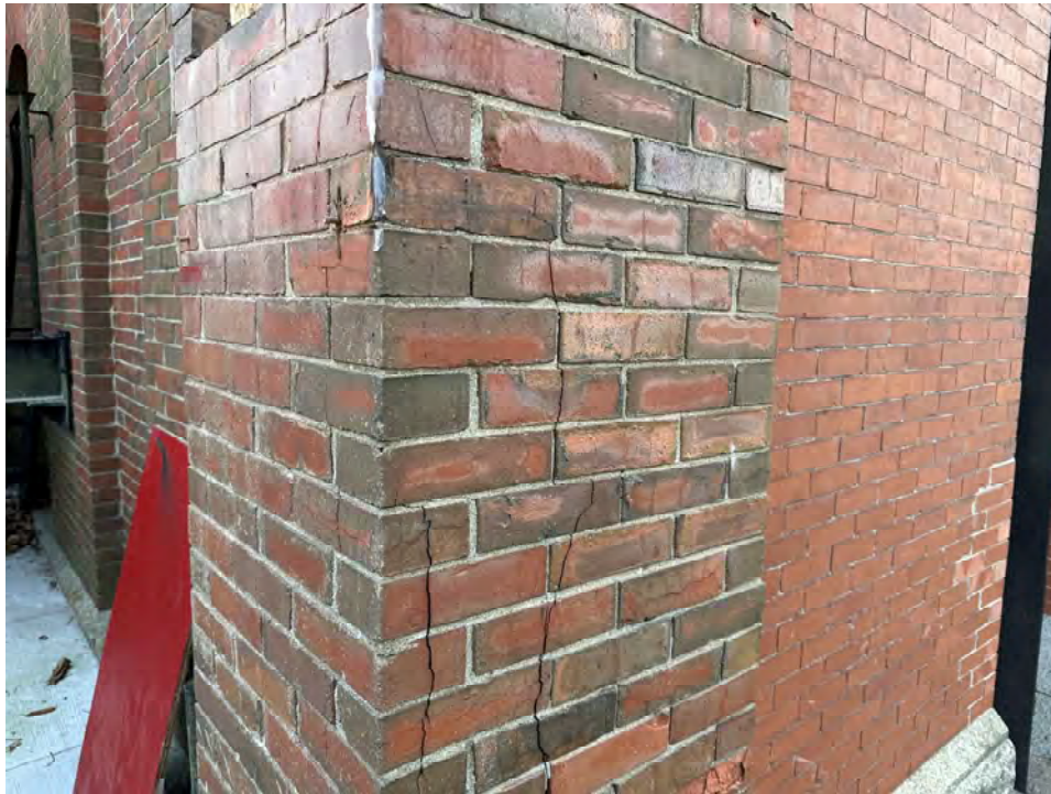
Photo 23: Close up of brick cracking and deterioration at northwest corner pilaster
