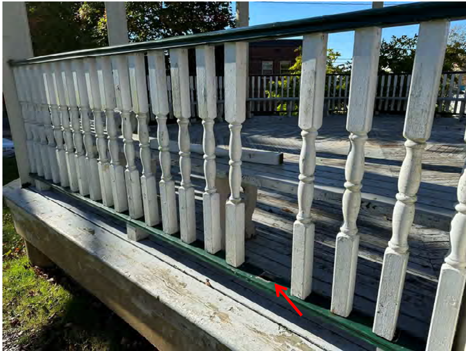
Photo 11: Section of guardrail with missing baluster
