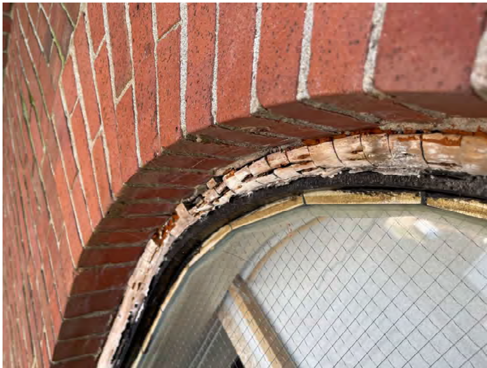
Photo 36: Peeling paint and deterioration of exterior wood detailing above retrofit vinyl window
