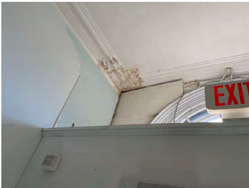
Photo 40: Moisture ingress deterioration above south elevation Cumberland Street entrance
