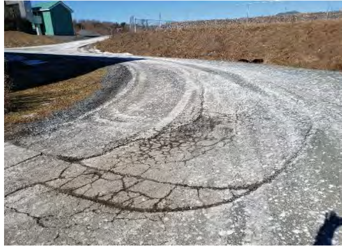
Access road to overhead garage door and rear of Process Building - localized settlement. Remove unsuitable base and reconstruct/patch roadway in 0-5 years.
