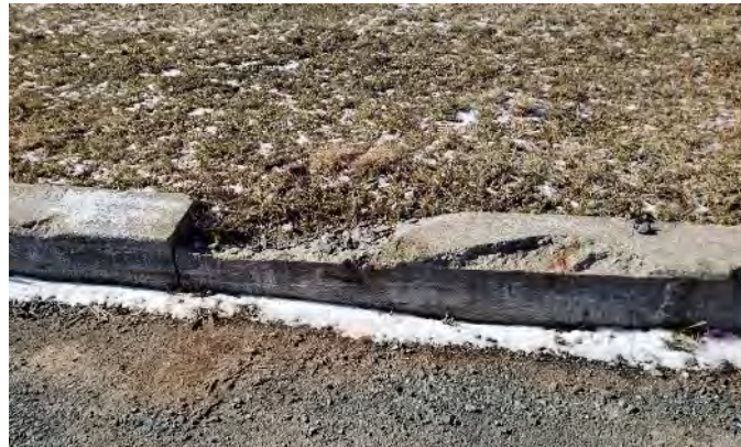
Impact-damaged high-back concrete curb. Replace damaged curb sections when access roads are resurfaced.
