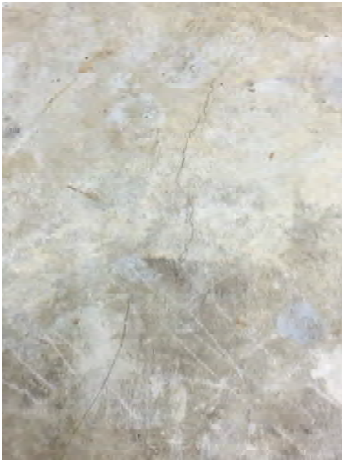
Cracks in floor slab of Process Room 112
