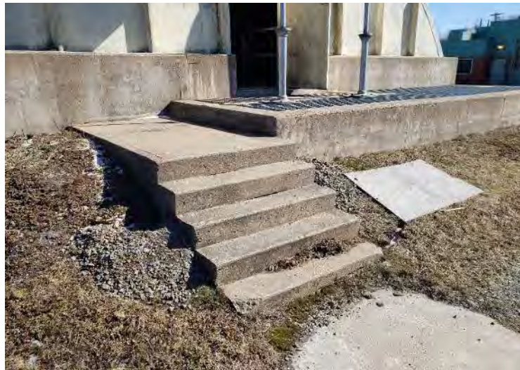
Bioreactor Building stairs; damaged corner.
