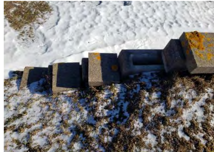
Missing retaining wall coping/cap section.
