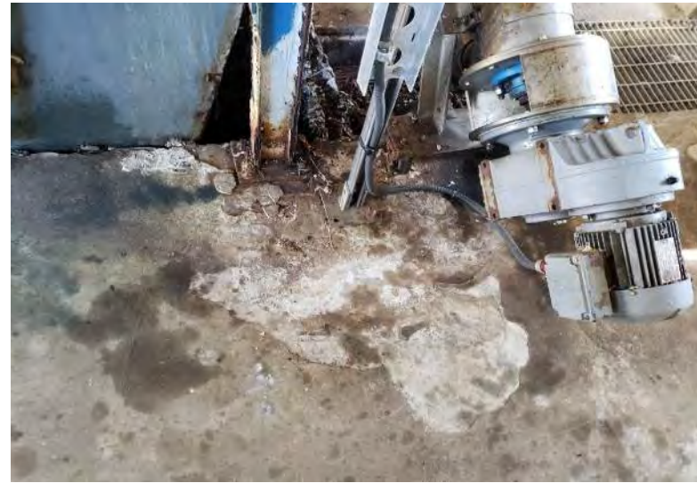
Surface scaling of concrete in the headworks area.
