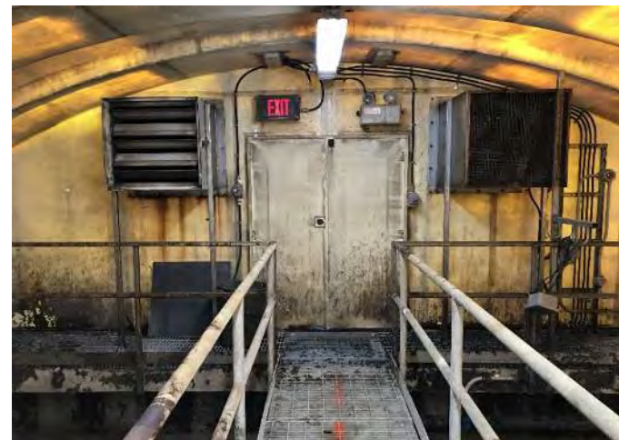
Intake and exhaust air ductwork (to the Biofilter Fan Building beyond ) in fair condition.
