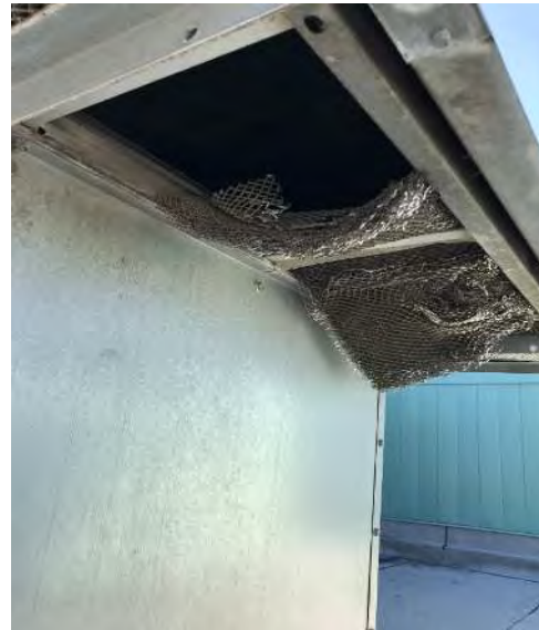
Supply Fan # 1 intake screens damaged and should be replaced.
