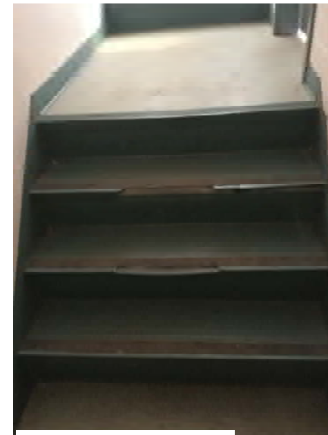
Torn nosing on stairs in Cooridor
