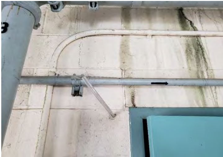
Typical step-crack at a re-entrant corner of masonry construction; headworks area door opening.
