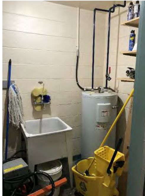
Electric water beyond its reliable service life.
