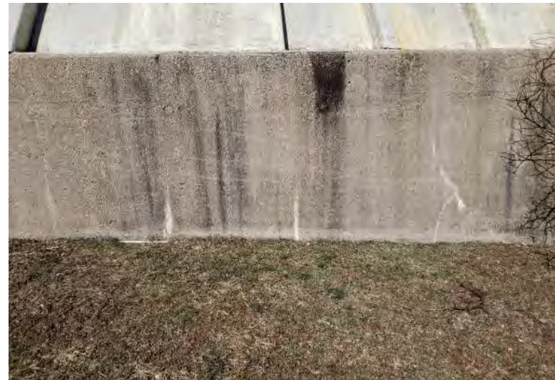
Close-up view of temperature and shrinkage cracks in the perimeter concrete walls of the Bioreactor Building
