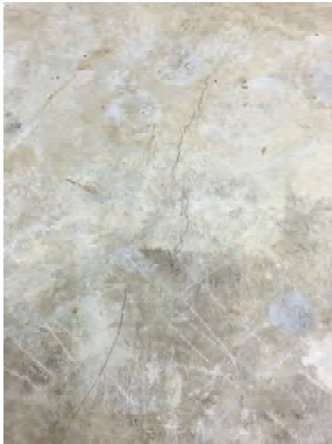
Cracks in floor slab of Process Room 112
