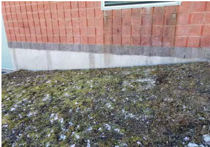
Minor temperature & shrinkage cracks in concrete foundation wall.
