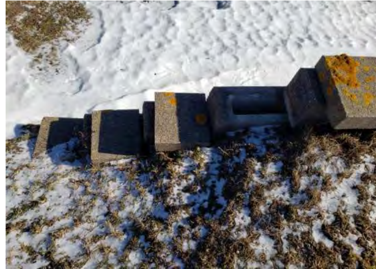
Missing retaining wall coping/cap section.
