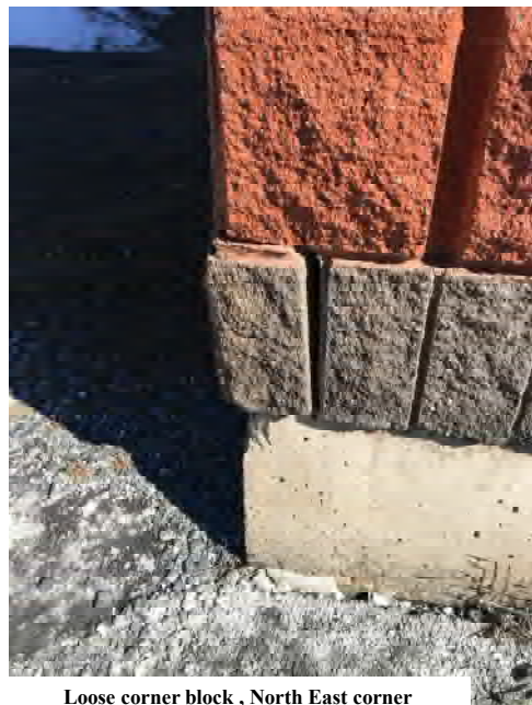
Loose corner block , North East corner of Process building
