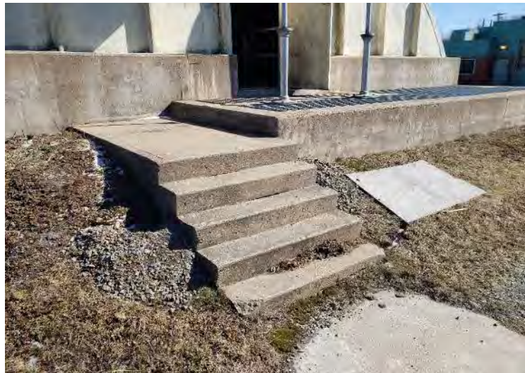
Bioreactor Building stairs; damaged corner.
