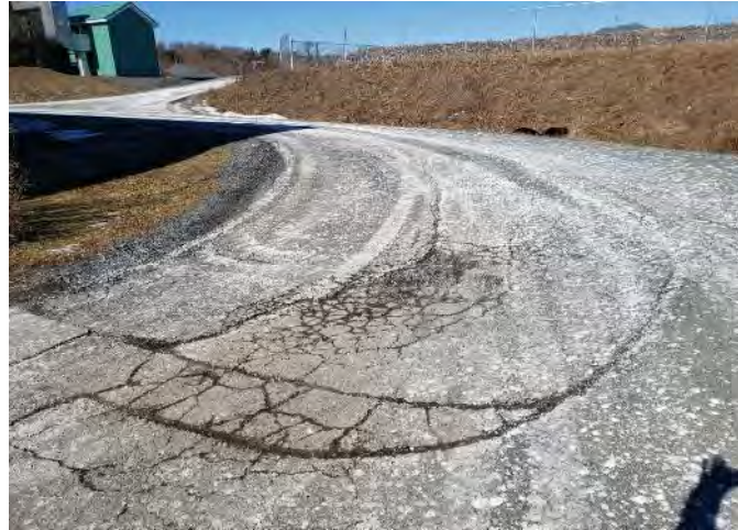
Access road to overhead garage door and rear of Process Building - localized settlement. Remove unsuitable base and reconstruct/patch roadway in 0-5 years.
