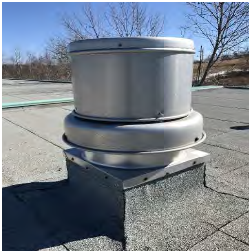
Typical original equipment exhaust fan on roof nearing end of reliable service life (EF-3 shown).
