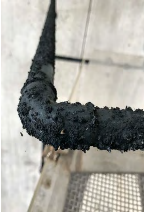
Typical corrosion and blistering paint on copper piping.
