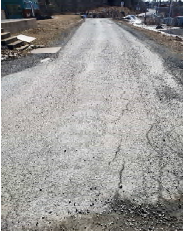
Bioreactor building access road - rutted and cracked. Repave in 5-10 years.
