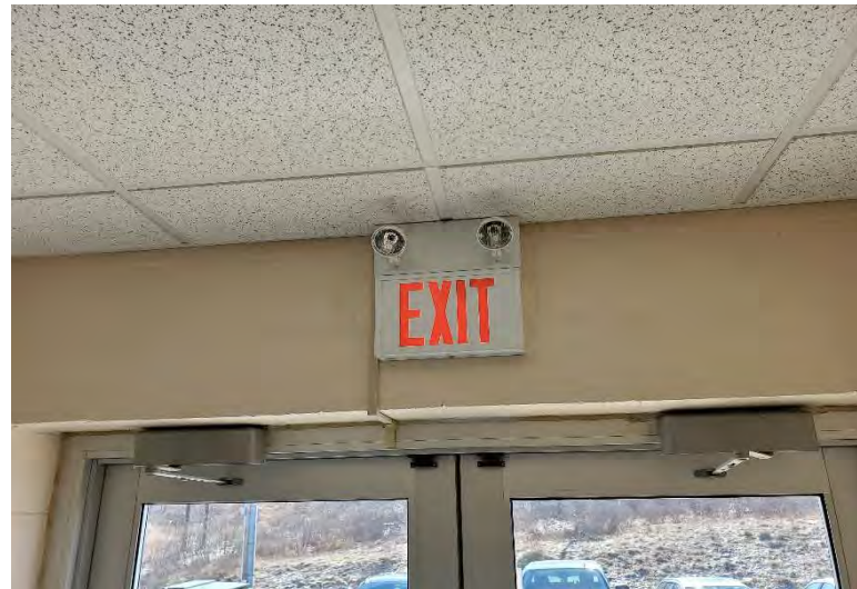
Suggest replacing red exit signs with newer green running man.
