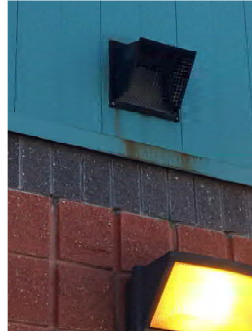
Staining and rust on metal siding under mech vent.
