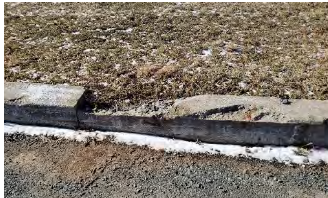
Impact-damaged high-back concrete curb. Replace damaged curb sections when access roads are resurfaced.
