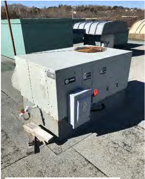
AHU serving office/lab to be replaced.
