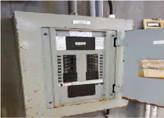
Panelboard in process area is very corroded.
