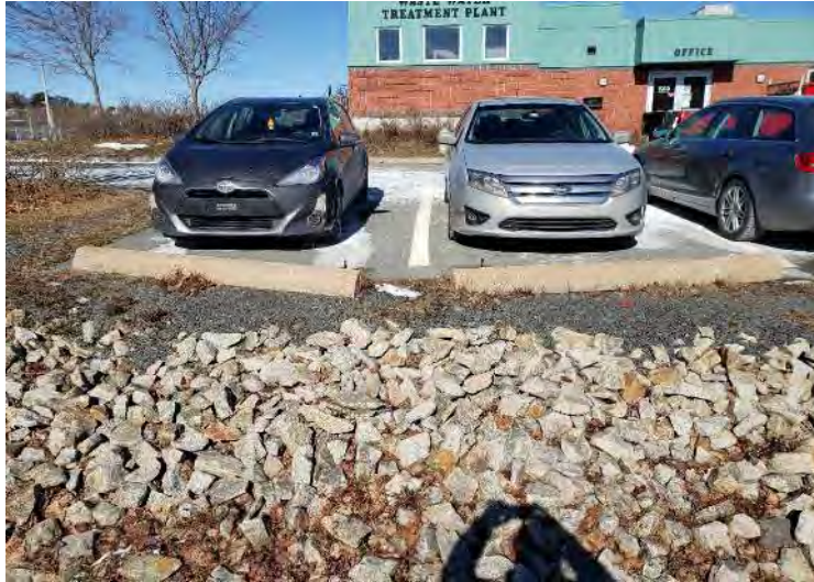
Precast curb sections dislodged from pins/dowels by apparent snowplow impact damage; it appears that the curb sections are undamaged and could be reinstalled.
