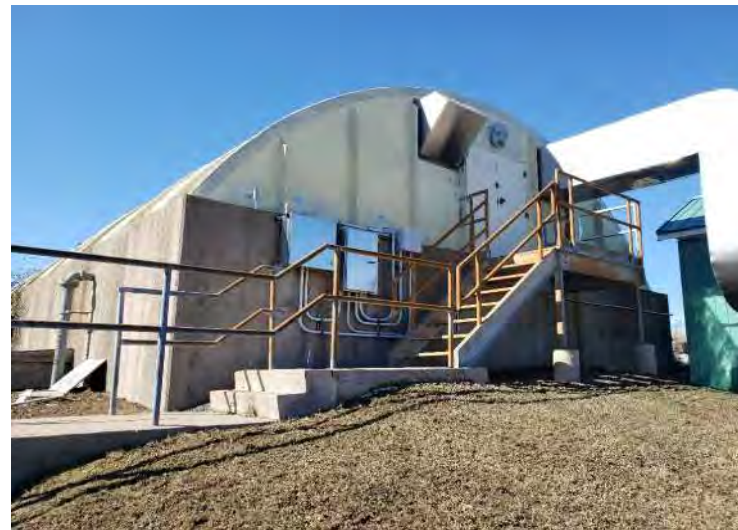
Bioreactor Building: surface rust on HDG stair assembly and railings.
