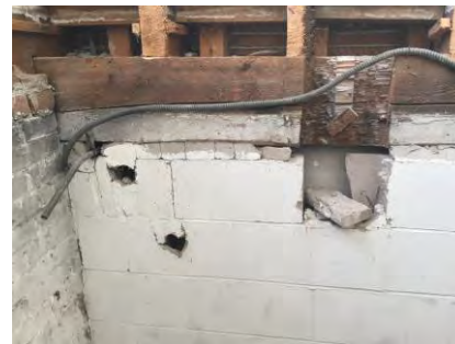
8. Damaged block to be repaired
