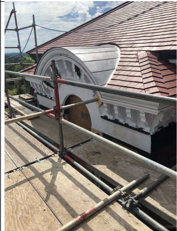
Figure 54 – Palladian windows to the south of the east elevation repaired and primed.
