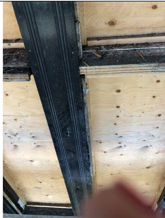
Figure 60 –Detail of transom sill loose connection to central trim due to previous interventions to the transom sills. In this case repair will preserve the transom sill.
