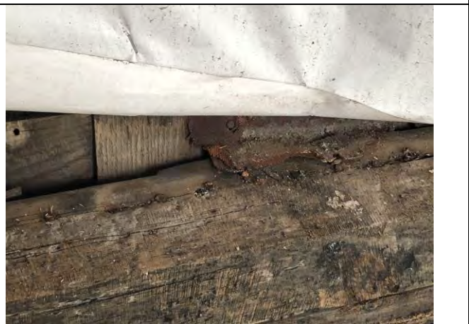
Figure 16 –rusted nails in woodwork created cracks and allows for water penetration. This is a case of wood element replacement with replica.
