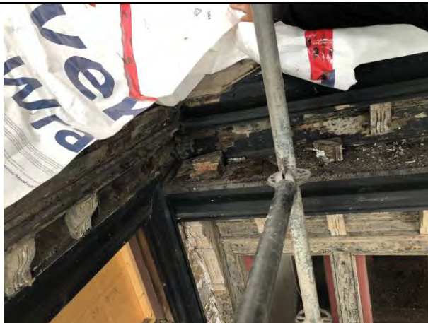
Figure 19 – Poor condition of woodwork at cornice. Most elements are rotten and are being repaired using dutchmen or replaces by replicas being made in the shop.
