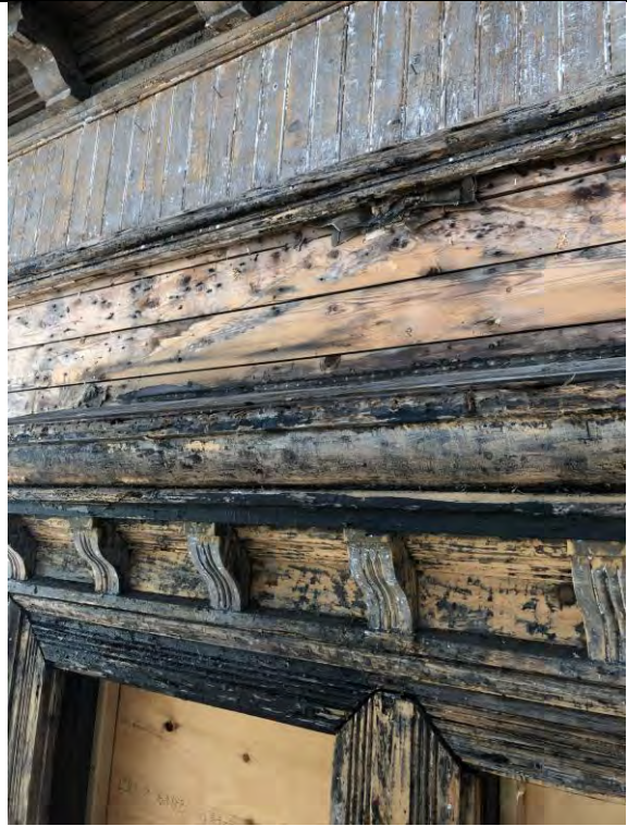
Figure 48 – Cornice above windows to be repaired.
