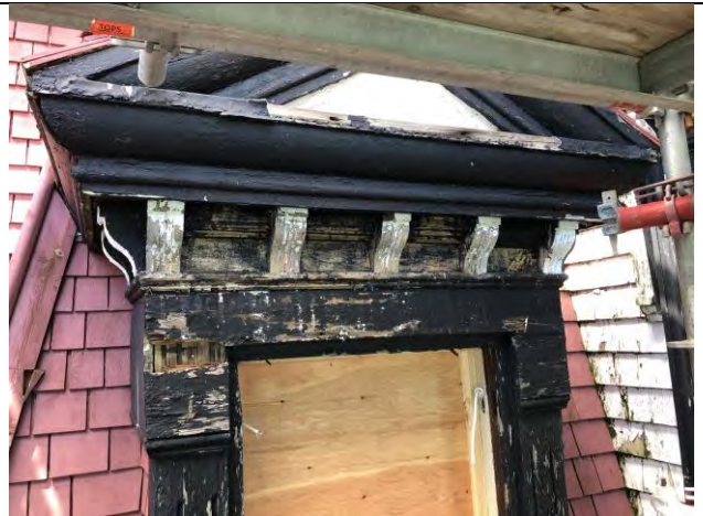
Figure 24– Detail of rotten wood at pediment and window woodwork.
