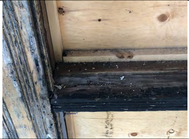
Figure 62 –Detail of transom sill, showing poor condition of rotten wood.
