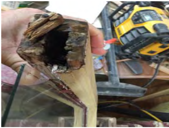
most decorative profile with poor mortice joint
