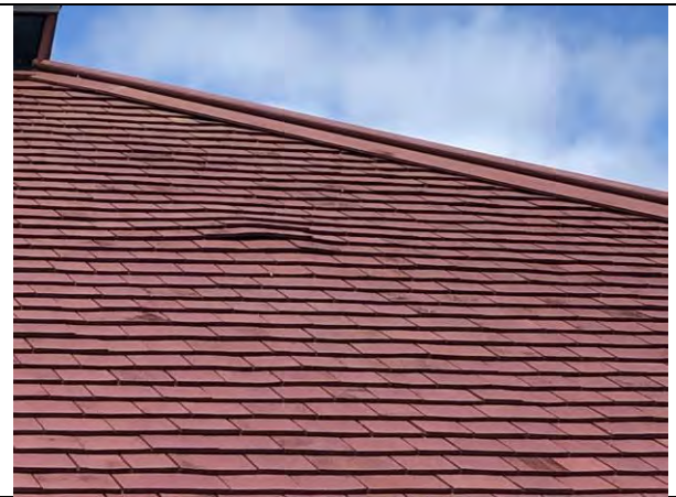
Figure 2- Zoom in- Visible deformation at the center of the roof,
