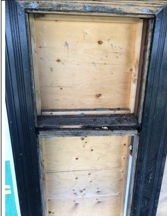
Figure 57 –Detail of transom sill, partially replaced in previous interventions.
