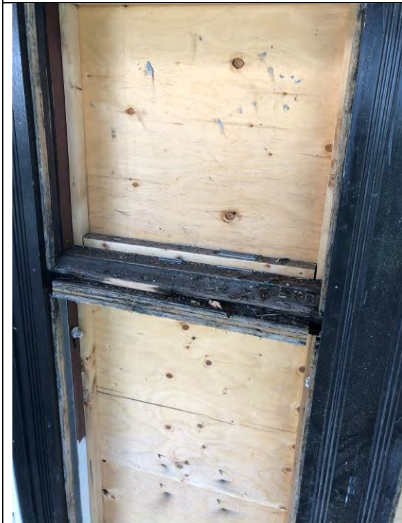
Figure 63 –Detail of transom sill, partially replaced in previous interventions.
