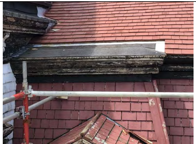
Figure 8 – Existing asphalt layers not replaced by Lead Coated Copper flashing
