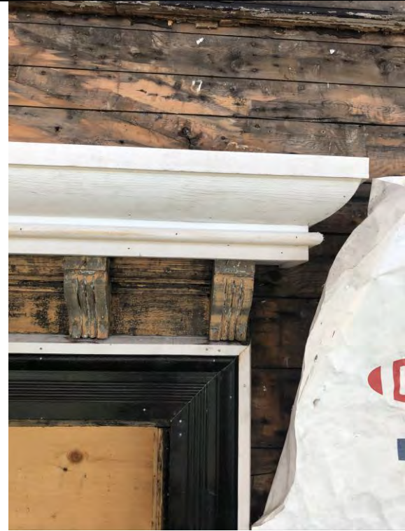
Figure 28– Pediment parts being replaced. Repaired trim with historically appropriate motif. Wood sheathing around window in good condition.
