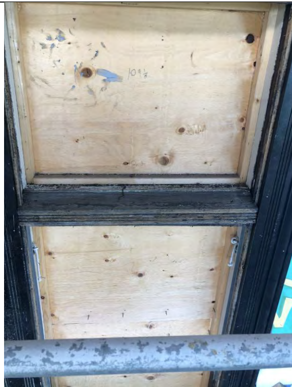
Figure 64 – Cracks in transom sills
