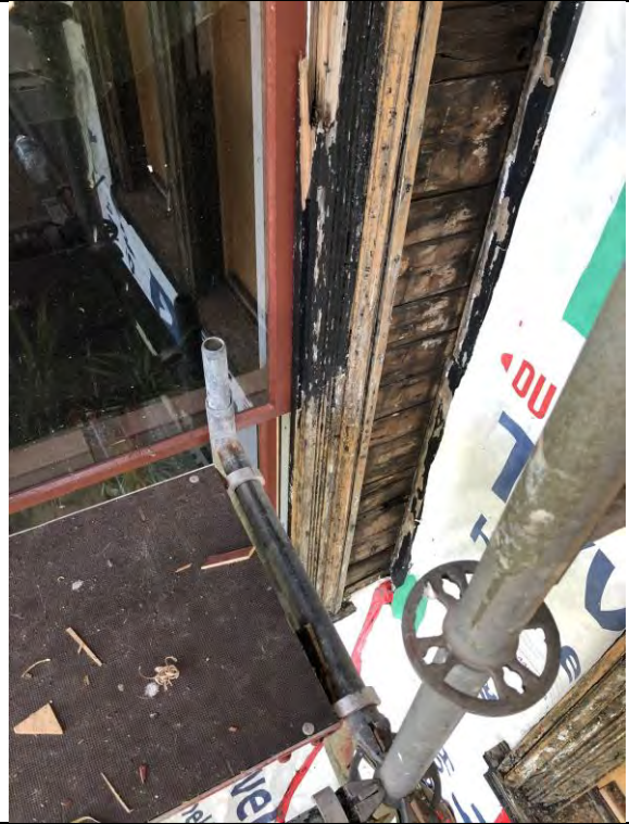
Figure 22 – Detail of rotten wood at trim.
