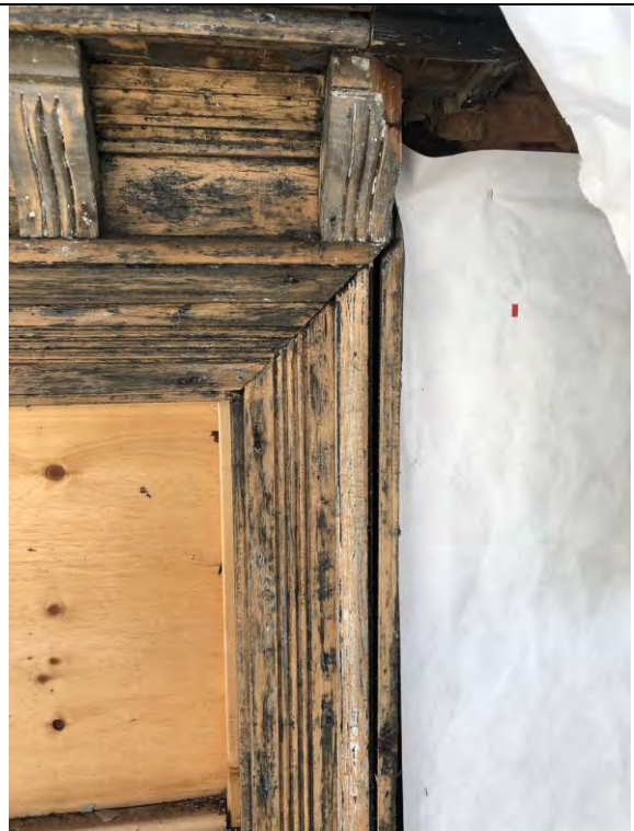
Figure 16 –Woodwork (corbel) at window requiring a dutchmen repair.
