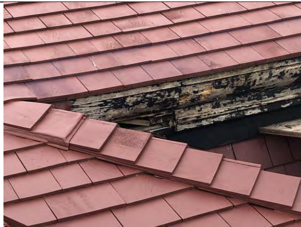
Figure 9 – Roof detailing at eaves to be completed after repair of wood eaves.
