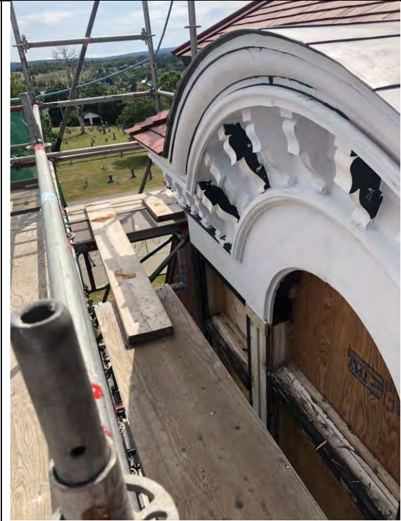
Figure 52 – Palladian windows to the south of the east elevation repaired and primed.
