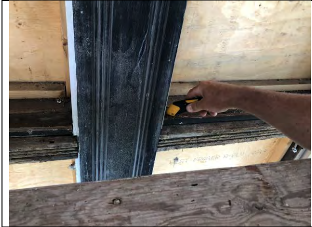
Figure 65 –Testing softness of wood at transom sill.
