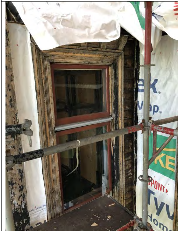
Figure 15 –Rotten wood discovered after paint removal at trims. Typical.
