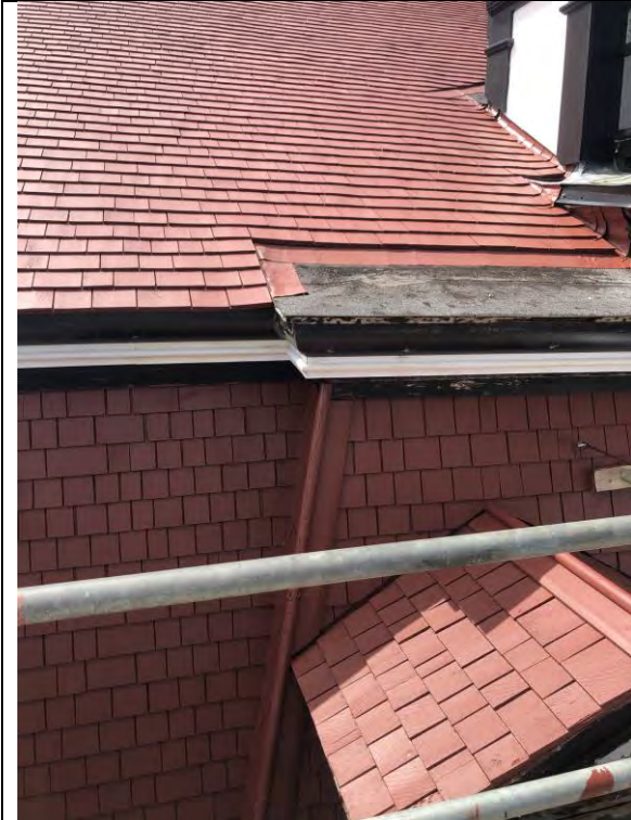
Figure 5- Asphalt on roof deck in fair to poor condition. Close view.
