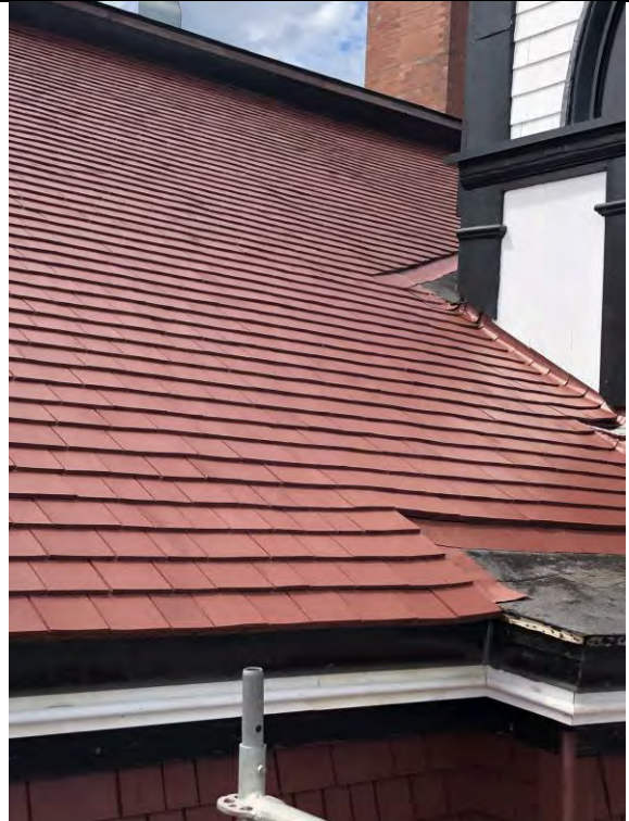
Figure 6- Roof shingle replacement completed. Asphalt on roof deck in fair to poor condition.
