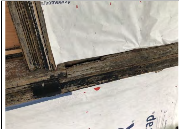
Figure 13 –Detail of sill partially replaced that is currently rot. In this case the sill will be replaced and connections between parts on weather exposed areas will be avoided.
