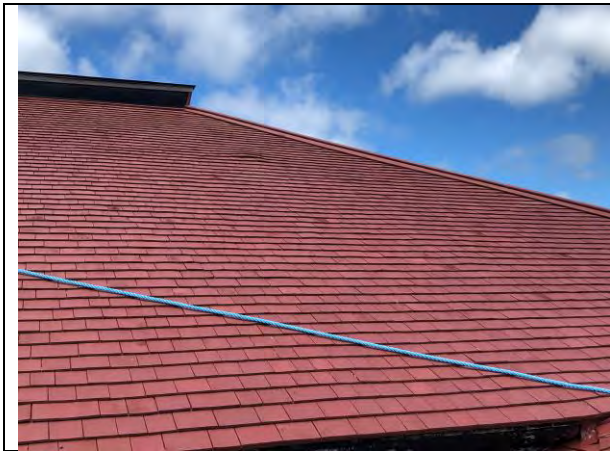
Figure 1- Re roofing: installation of new shingles close to completions. Visible deformation at the center of the roof.
