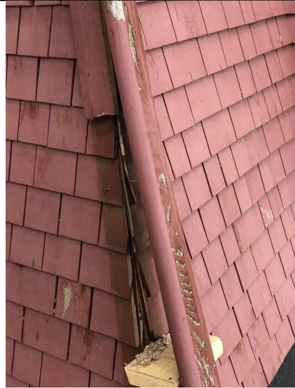
Figure 8 – Cladding on the 3 rd floor that is being repaired. Roof hip cap to be replaced.
