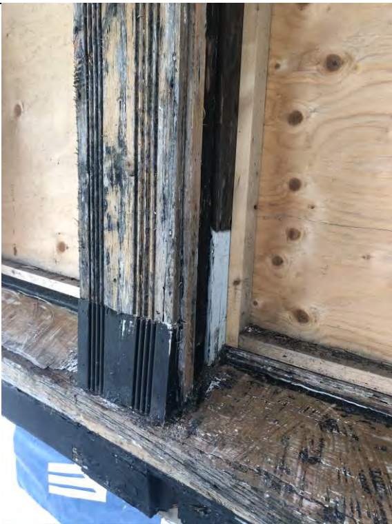
Figure 25 – Previous inappropriate repair to be removed.
