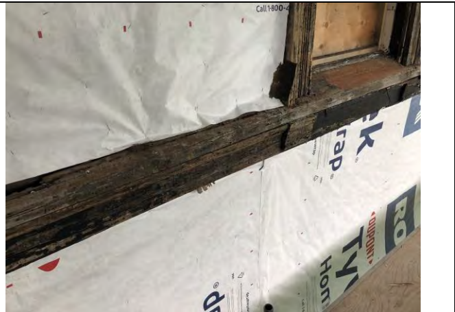
Figure 14 – Rotten wood at band between sills. Typical.
