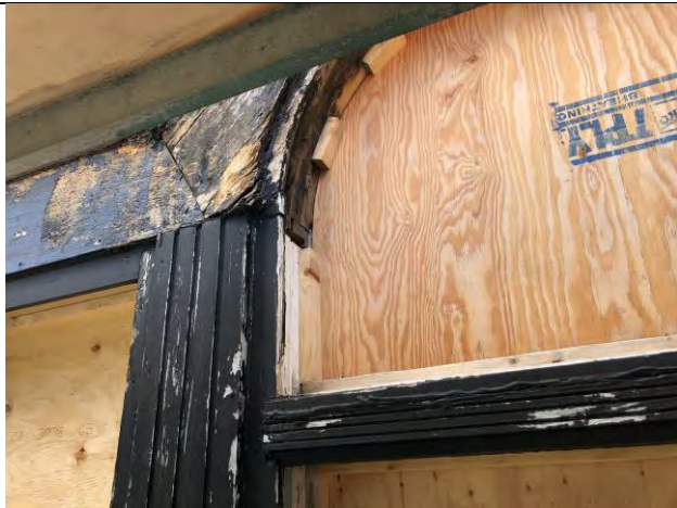
Figure 23 – Detail of rotten arched window.
