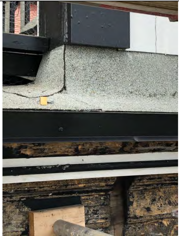
Figure 12- Asphalt on the top of the cornice on the bell tower.
