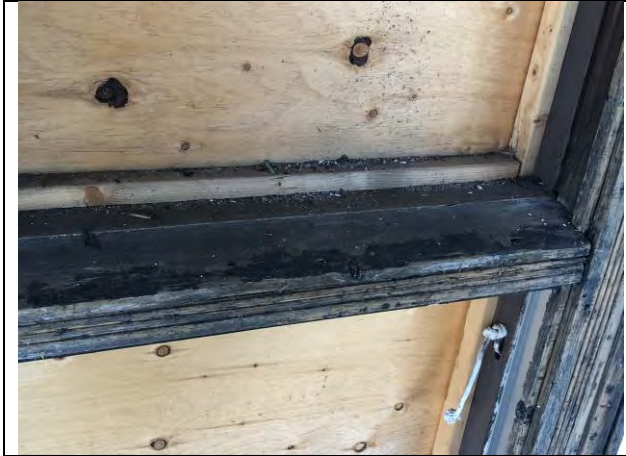
Figure 61 –Detail of transom sill, showing previous interventions.
