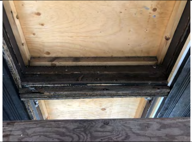
Figure 66 –Detail of transom sill to be replaced.
