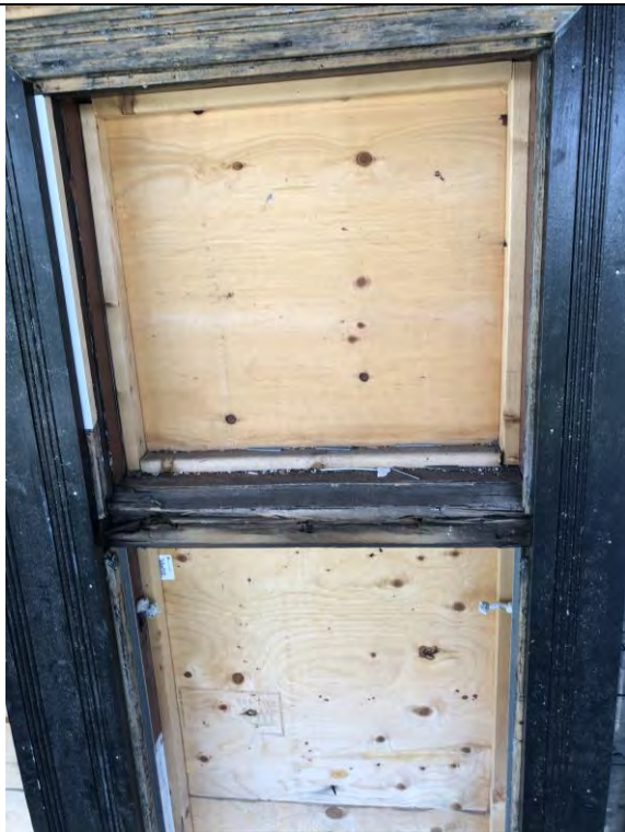
Figure 59 –Detail of transom sill, partially rot.
