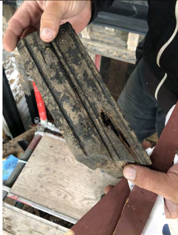
Figure 22 – Detail of wood in fair condition to be prepared and reused at same location.
