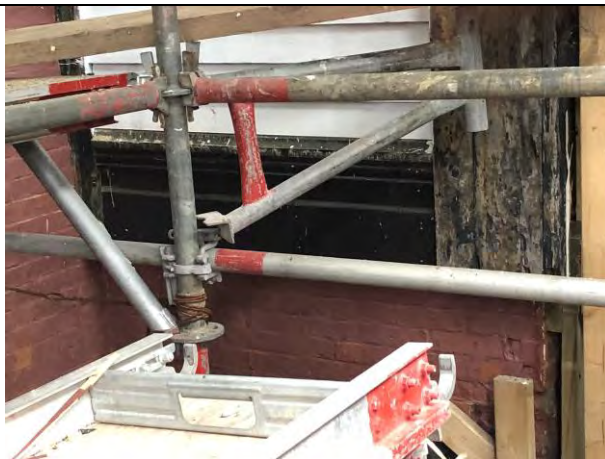
Figure 23 – Detail of water table at the ground level to be replaced.
