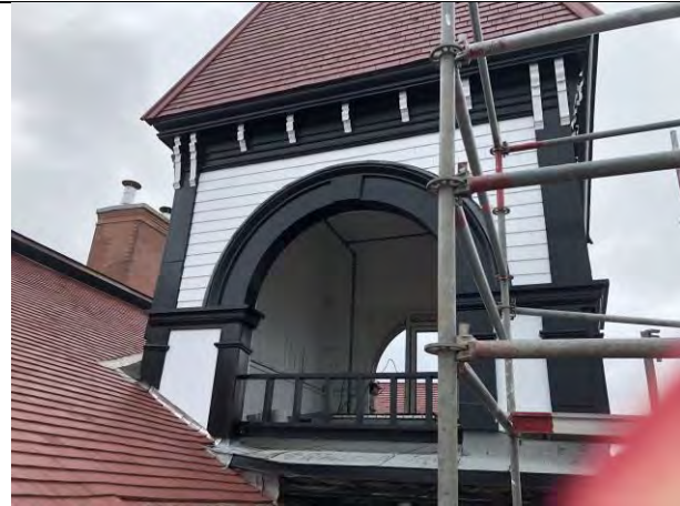
Figure 5 – Bell tower. The bell is removed, and a metal net is installed to prevent birds entering the tower.
