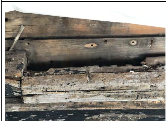
Figure 15 – Detail of rotten sill previous repair. Part of the element is lost.
