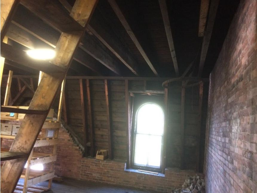
Photo 11 – Rafters for the Mansard-style portion of the roof of the south section of the building
