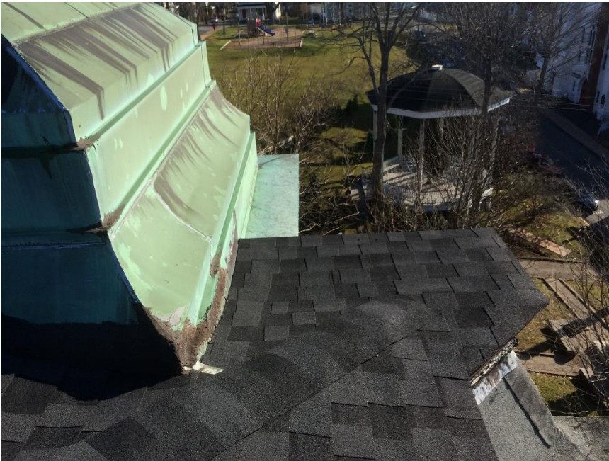
Photo 18 – Water-damaged shingles (2 of 2)
