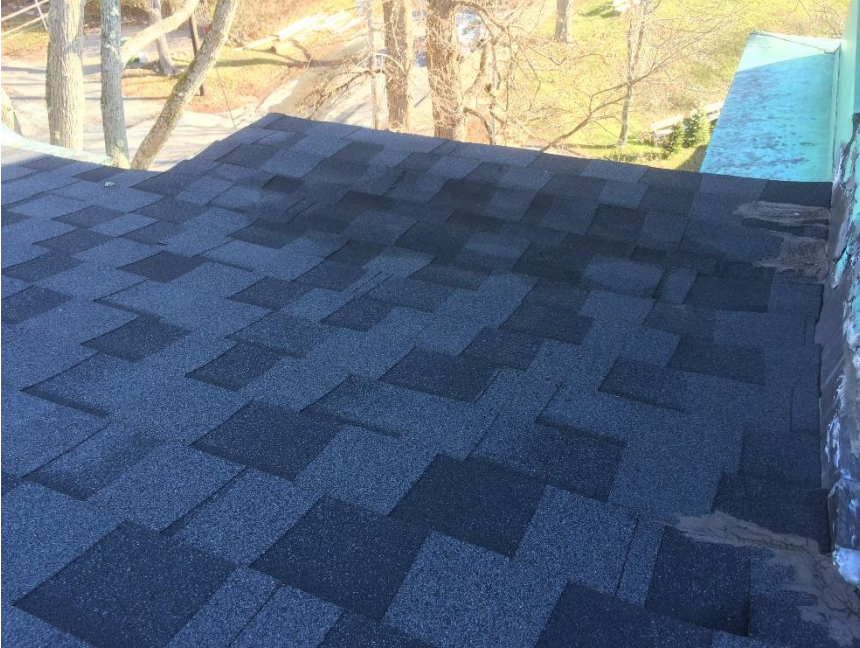
Photo 17 – Water-damaged shingles (1 of 2)
