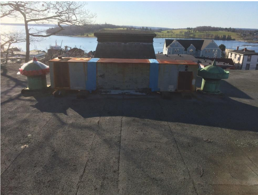
Photo 8 – Rooftop mechanical equipment
