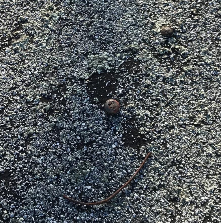
Photo 21 – Screw in roof membrane (1 of 2)
