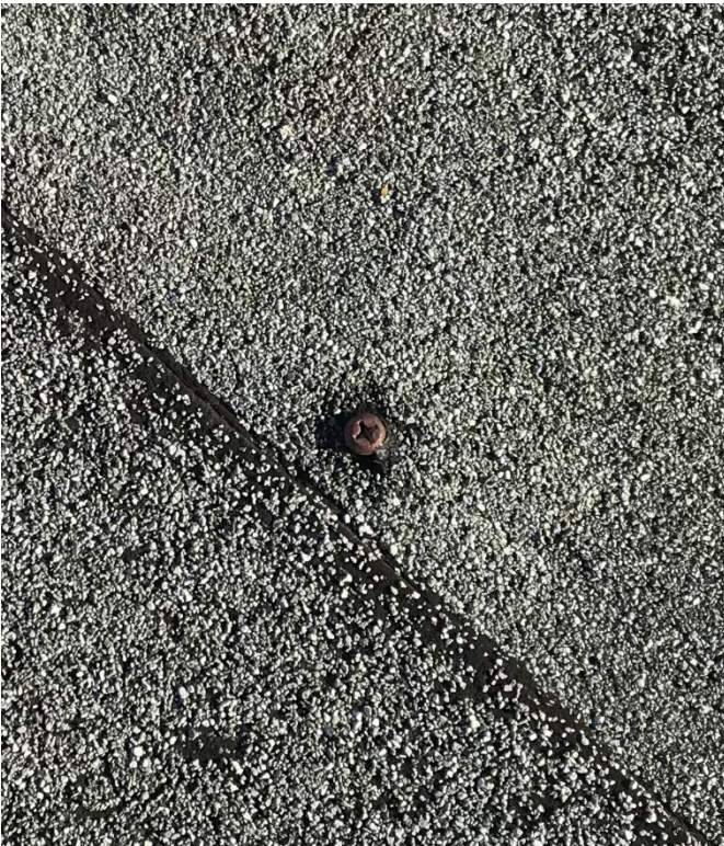
Photo 22 – Screw in roof membrane (2 of 2)
