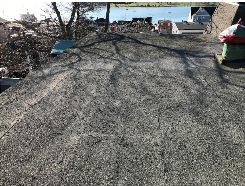
Photo 20 – Moss growth on roof membrane
