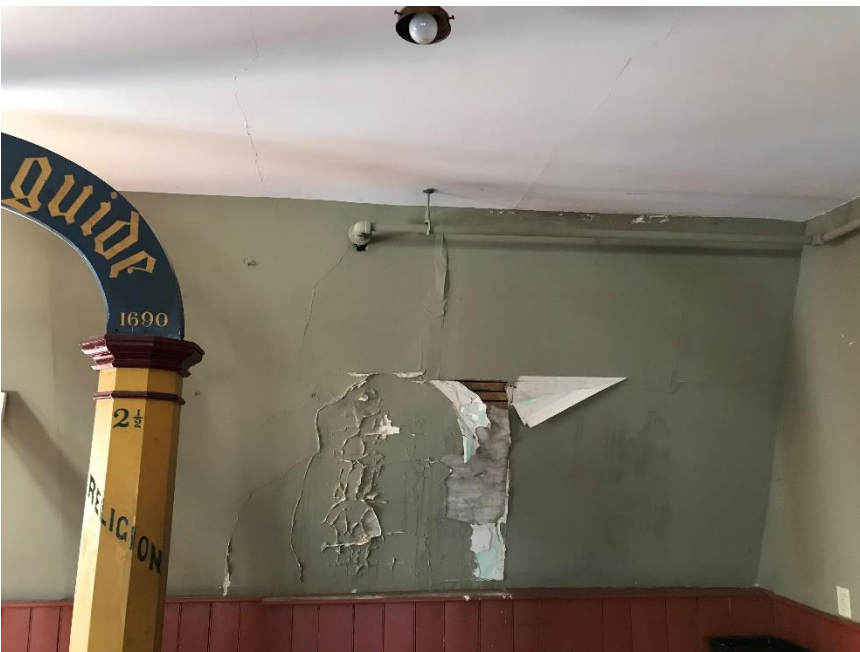
Photo 40 – Interior water damage (2 of 3)
