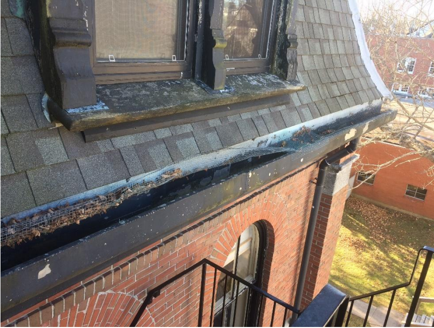
Photo 37 – Bent steel mesh above gutters
