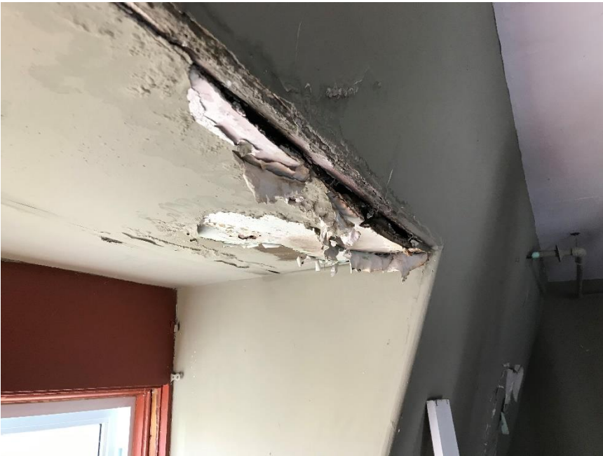
Photo 38 – Interior water damage, typical around dormers
