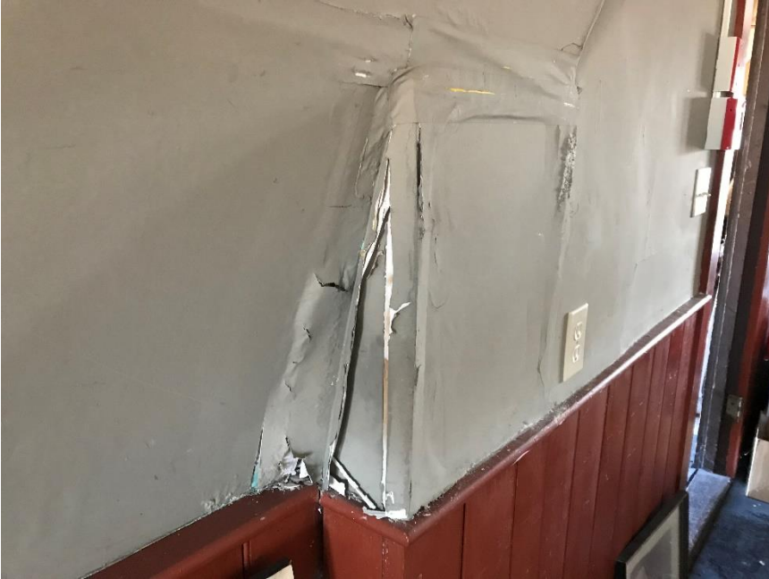
Photo 41 – Interior water damage (3 of 3)
