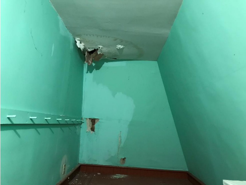
Photo 39 – Interior water damage (1 of 3)
