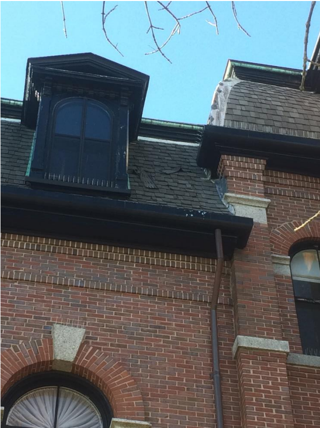
Photo 19 – Damaged shingles on Mansard-style roof (west side of building)
