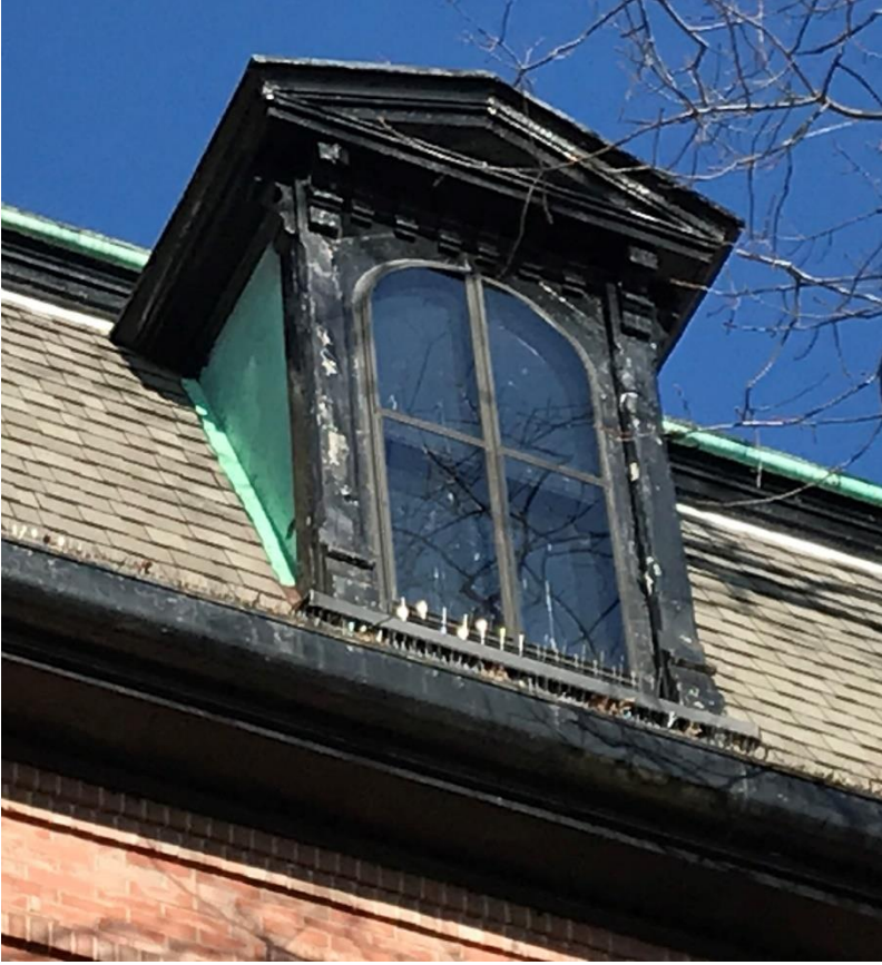
Photo 25 – Paint peeling from wood trim on dormer
