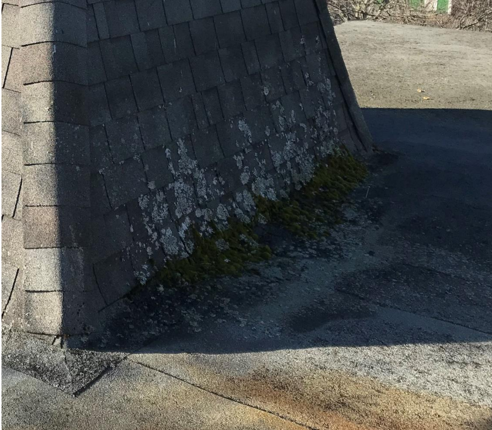
Photo 29 – Moss and lichen growth at base of former clock tower
