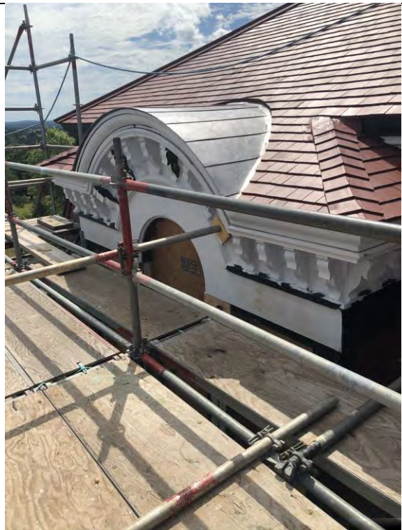
Figure 54 – Palladian windows to the south of the east elevation repaired and primed.
