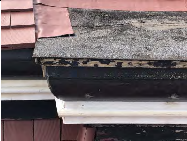
Figure 7- Asphalt on roof deck in fair to poor condition. Note the exposed and partially rotten wood deck underneath
