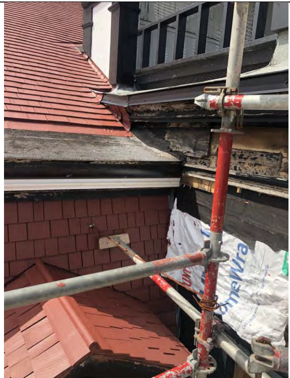
Figure 4- Shingles on mansard roof window on the 3 rd floor is completed. Asphalt on roof deck in fair to poor condition.
