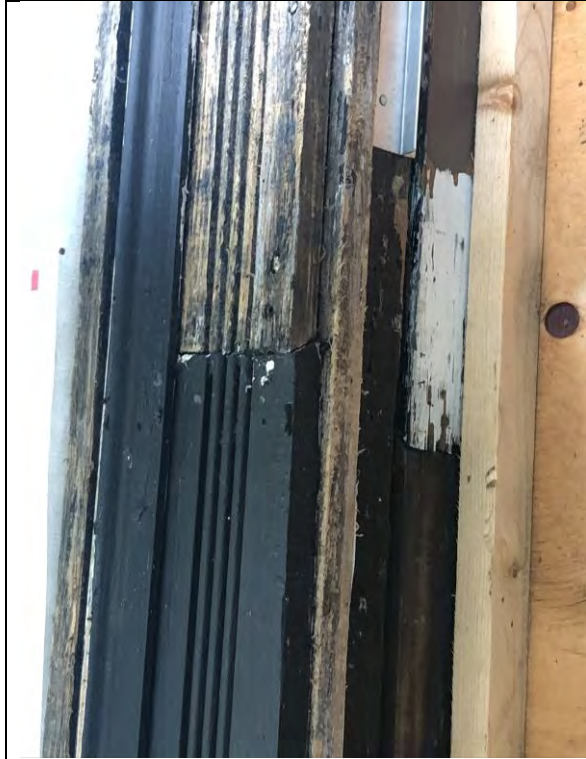
Figure 27 – Detail of existing repair with different and not historically correct decorative motif.
