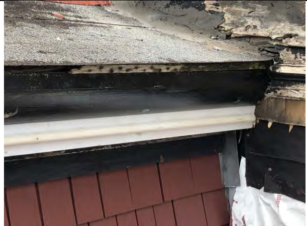
Figure 8- Asphalt on roof deck in fair to poor condition. Note the connection to the tower.
