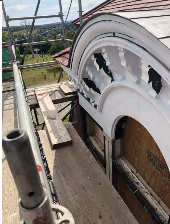
Figure 52 – Palladian windows to the south of the east elevation repaired and primed.
