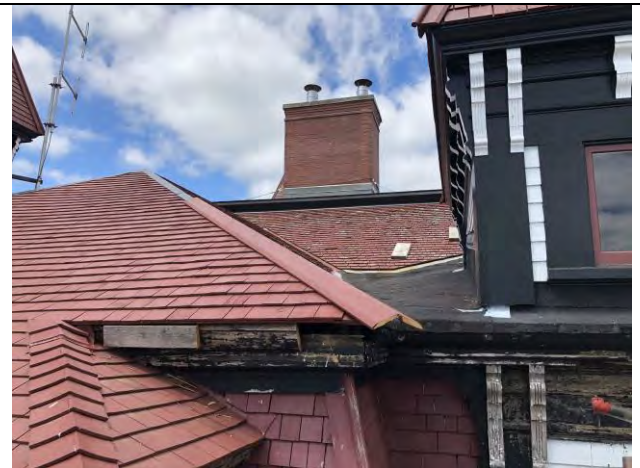
Figure 4 – in the center of the photo: area of roof to be re-shingled
