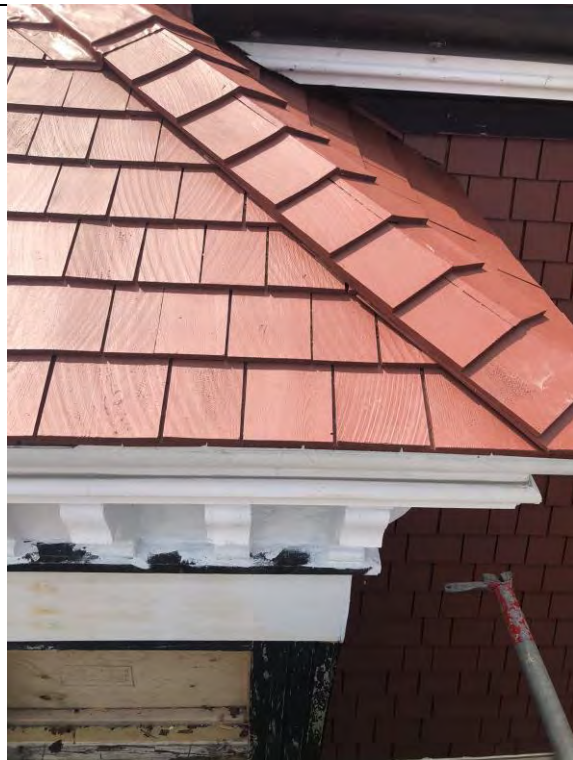
Figure 53 – Palladian windows to the south of the east elevation repaired and primed. Detail of the north corner.
