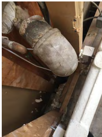
7. Existing piping & radiator
