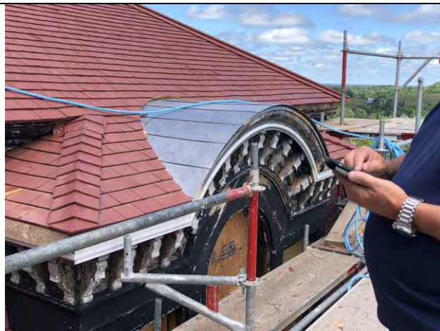
Figure 7 – Lead coated copper flashing on the barrel vault on windows E18, E19, E20.
