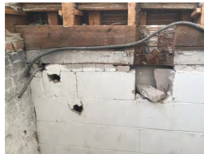
8. Damaged block to be repaired
