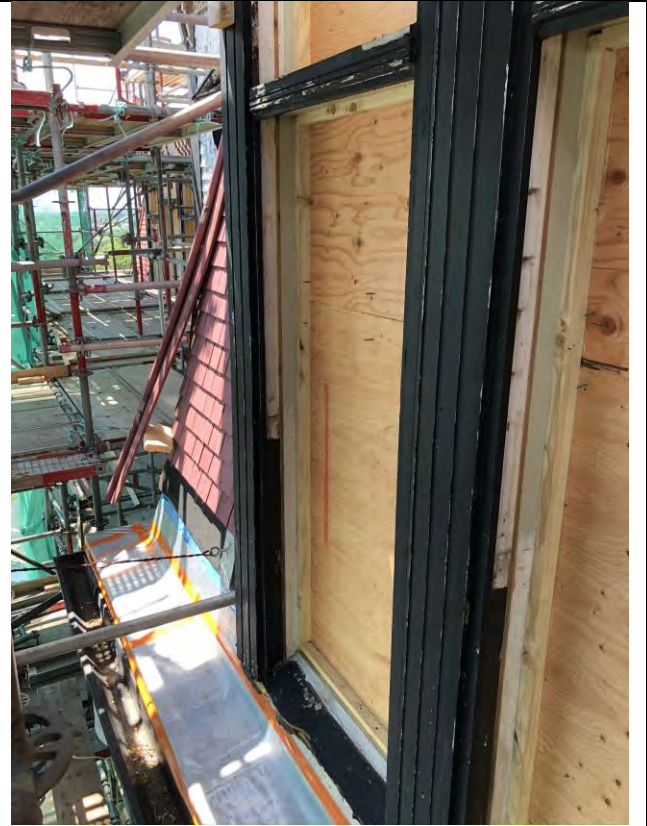
Figure 12 Protection in place on the top of the cornice, between 2 nd and 3 rd level.
