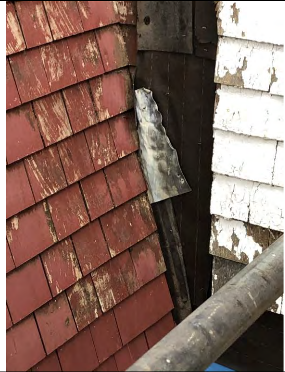
Figure 2- Detail of moss growth and existing temporary flashing at the connection between cladding and roof to the left of window E15.
