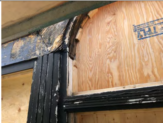
Figure 23 – Detail of rotten arched window.
