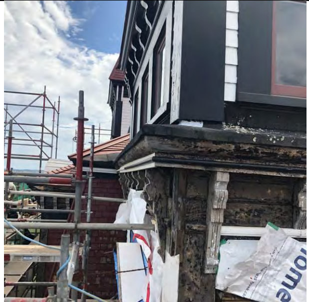
Figure 10- Asphalt on the top of the cornice on the north tower. Corner.
