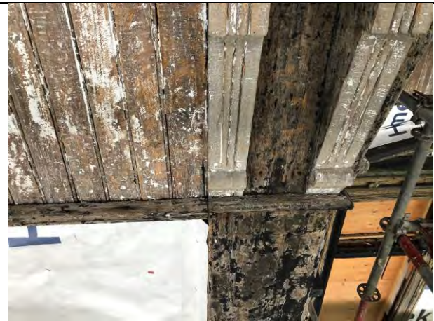
Figure 10– Siding on the 3 rd floor elevation- paint is removed. Wood is in good condition.
